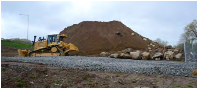
NO Stockpiling of Excavated Materials
