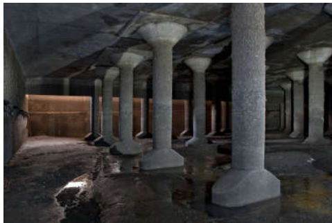
Toronto: Keelesdal-Hyde Ave Underground CSO Storage Tank
