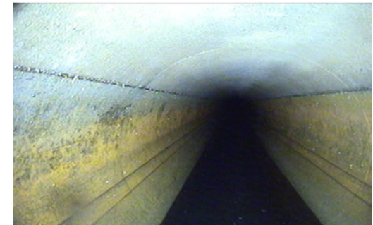
Maximize use of the collection system for storage
