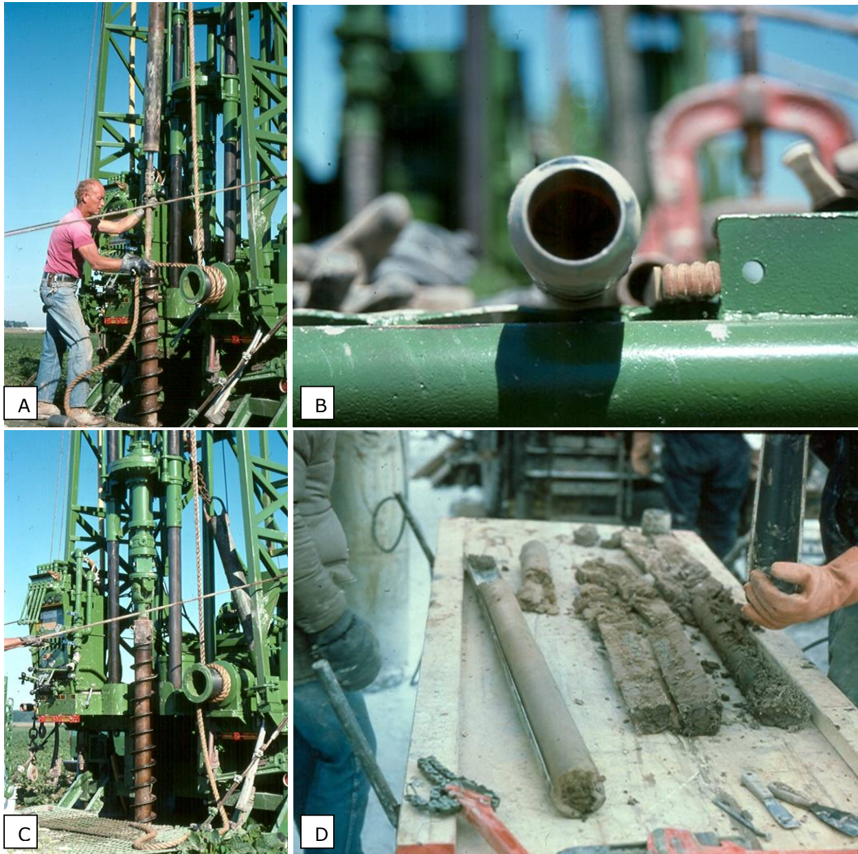
Figure 1-12. These images illustrate a typical geotechnical boring operation using hollow-stem augers. The rig pictured here is on the large side, capable of drilling to depths of 100 feet or more. A) a 140-lb hammer, represented by the cylinder on the drill rod above the operator's hand, falls 30 inches, driving a split spoon coring device into the sediment. The number of blows required to advance the split spoon one foot is a standard measure of hardness ("N" value, or blow count) recorded for every borehole; B) the business end of the sampling barrel, which can range from 18 inches to 5 feet in length, and 1 to 4 inches in diameter, depending on the objectives of the project and the level of detail needed. For routine geotechnical investigations, one 18-inch sample is typically taken in every 5-foot depth interval. More complex geotechnical investigations and environmental sites often require more frequent sampling; C) once the sampler has been retrieved from the hole, the augers are used to drill through the just-sampled interval. The process then repeats; D) the split spoon is separated, revealing a continuous core of sediment from the sampled interval, at least under ideal conditions. A number of problematic geologic conditions, such as large stones, heavy gravel, and runny, wet sand can lead to incomplete sample recovery. Photos by Tony Fleming.
