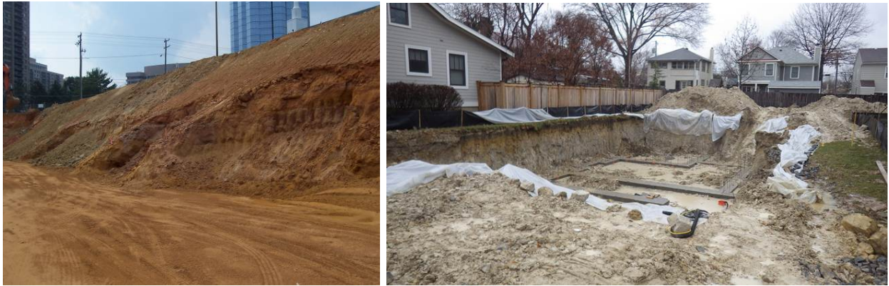
Figure 1-3. Excavations of various sizes can yield extremely valuable information about both local and regional geology, but they tend to be rather short lived, so timing is everything. The foundation excavations pictured above represent "holes of fortune" encountered during this project: a high-rise on King Street (left) and a much smaller house foundation in Del Ray (right). Unfortunately, thousands of other excavations made over the years in the City were never documented by a geologist or geotechnical engineer, so any useful information they might have yielded is lost. Photos by Tony Fleming (left) and R.H. Simmons (right).
