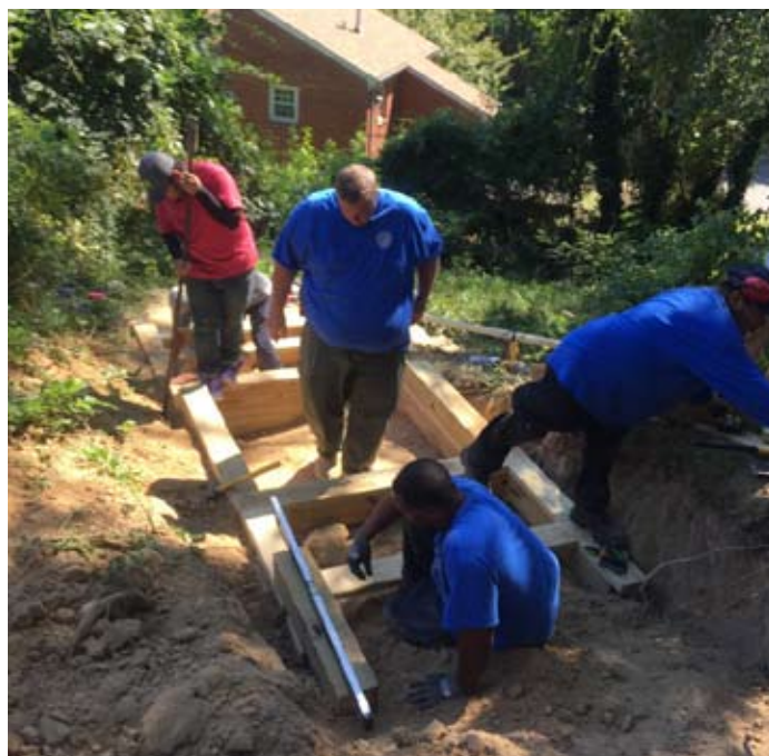
RPCA and ARHA Staff worked together in September 2015 to repair the stairs from the ARHA site to Mulligan Park.
