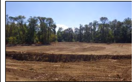
Freshwater Tidal Wetlands restoration area ready for planting at Four Mile Run Park.
