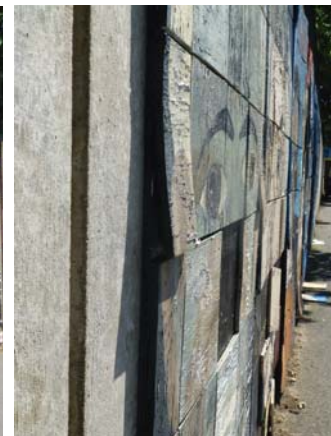
Figure 25. The plywood panels have warped.
