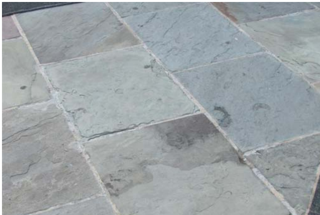
Figure 33. Slate pavers exhibit minor flaking and mortar loss typical to a highly-trafficked surface.
