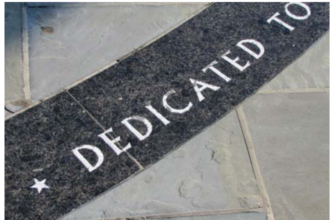
Figure 34. Paint is flaking from within the lettering on the inscribed granite pavers.
