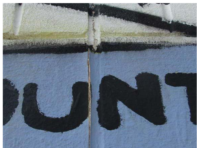
Figure 78. Paint is failing where it was applied over flexible sealant along an expansion joint.
