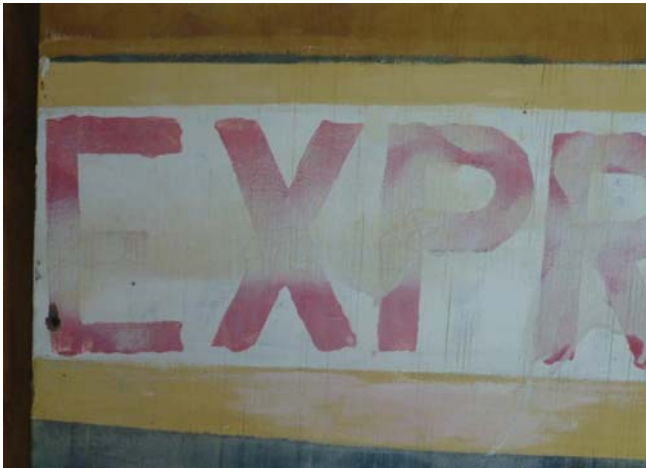
Figure 86. Graffiti spray-paint was observed in select locations.
