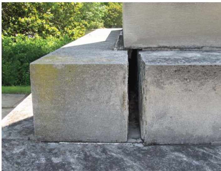
Figure 8. One of the limestone blocks that comprise the tiered base is displaced at least 2".
