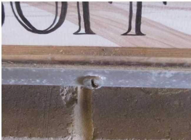
Figure 51. Minor pitting and corrosion of aluminum frame and fastener.
