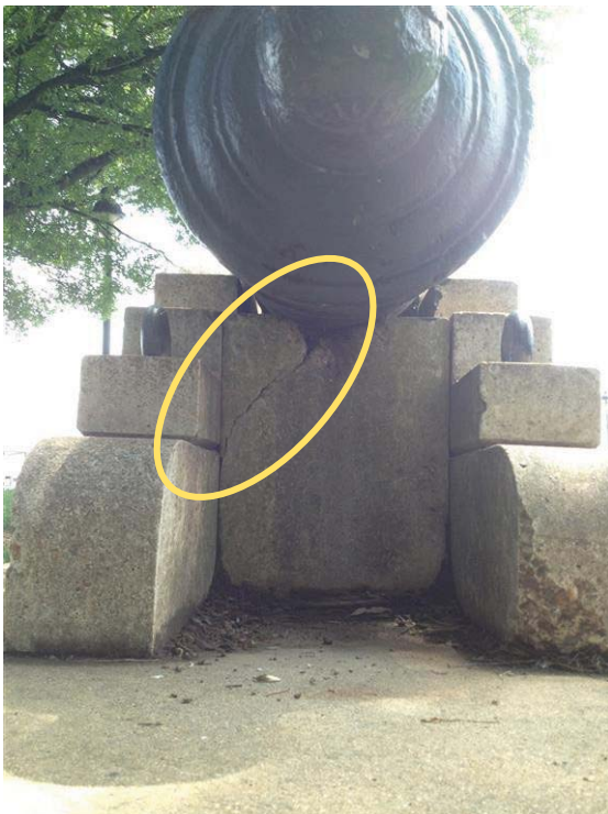
Figure 41. The concrete carriage has cracked and exhibits dimensional losses, suggesting the cannon may not be sufficiently supported.
