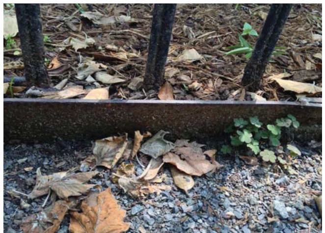
Figure 58. Steel bed liners and the fencing exhibit corrosion.
