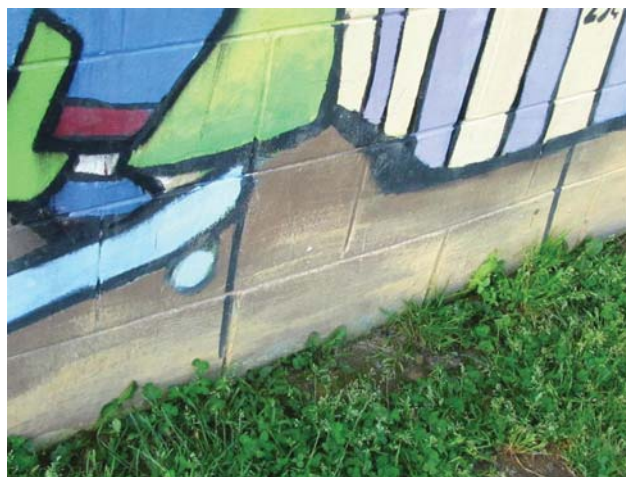
Figure 77. Splashback from the ground below has soiled the lowermost 12" of the mural
