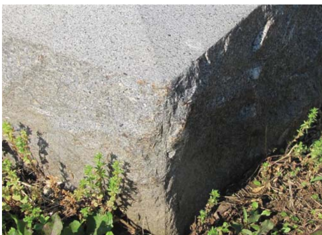
Figure 121. Iron staining on the edge of the plinth suggests abrasion from a lawnmower
