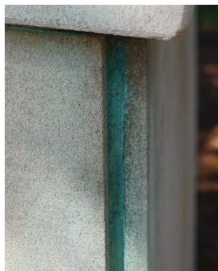
Figure 19. Copper staining has discolored the joints.
