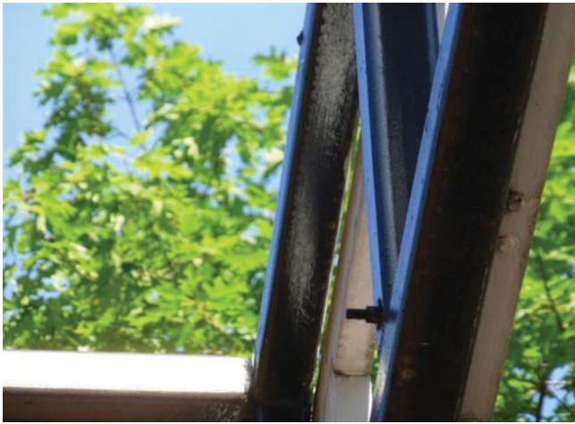
Figure 65. Bolts through the trellis introduce a potential point of weakness and allow water to impact the metal.
