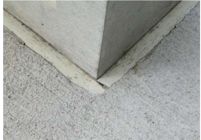
Figure 16. Detail of rigid plastic sealant, embedded around the base of a pillar.
