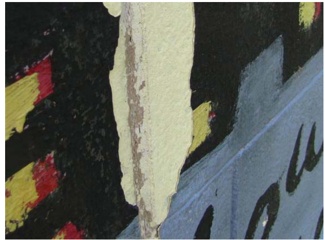
Figure 74. Peeling paint along the vertical expansion joint.
