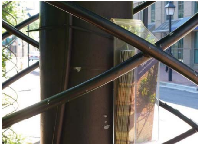
Figure 68. Zip ties have been used to affix brochure holders to some of the trellis posts, causing abrasion of the paint.
