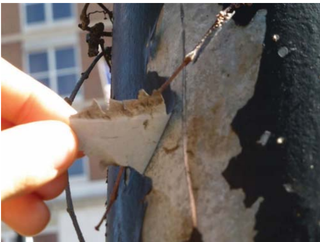
Figure 69. Detail of primer and topcoat peeling away from the galvanized steel surface.
