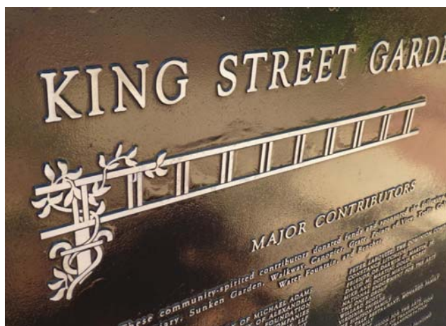
Figure 63. The painted background of the contributors' plaque is bubbling in select locations.
