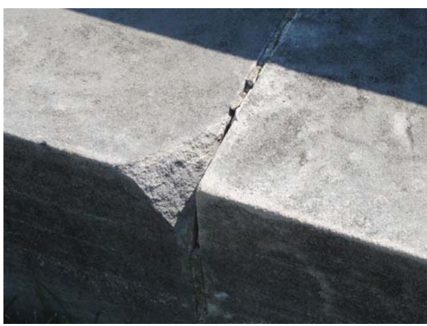
Figure 12: Typical limestone spall along an exposed edge.
