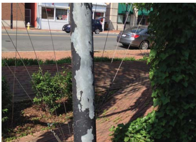
Figure 61. Typical paint loss on a steel structural member revealing the galvanized surface below.
