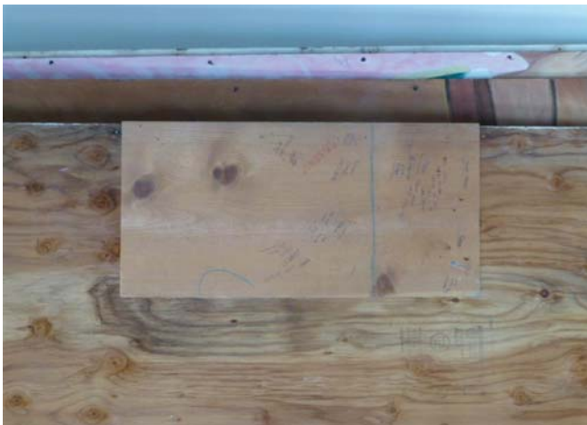
Figure 88. Wood blocking on the reverse of a panel used to support one of the major patching repairs.
