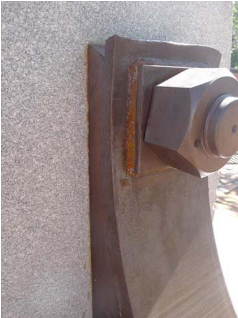
Figure 92. Corrosion and iron staining at the juncture where the steel flange meets the granite totem.
