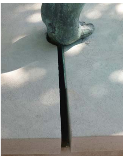
Figure 18. The coping stones of the pedestal have become displaced.
