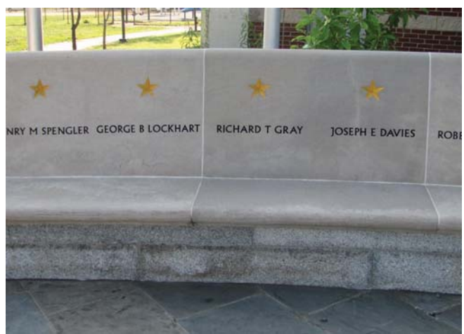
Figure 36. Staining and discoloration is typical of the granite blocks under the limestone bench.
