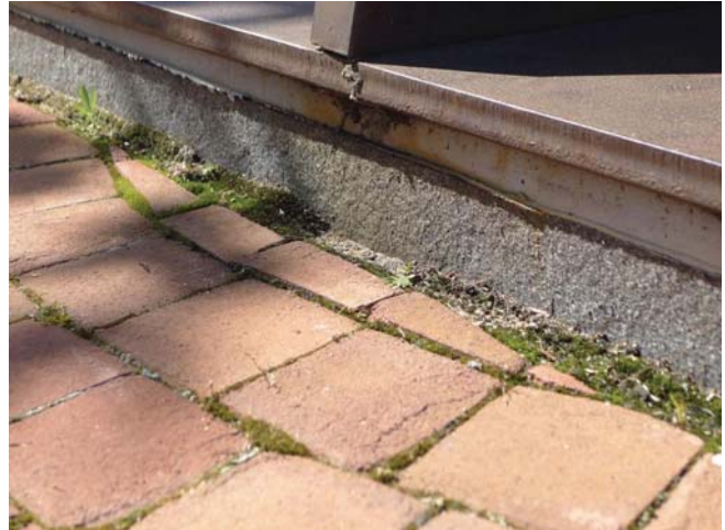
Figure 93. Iron staining of the granite base and vegetative growth in the pavers abutting the sculpture.
