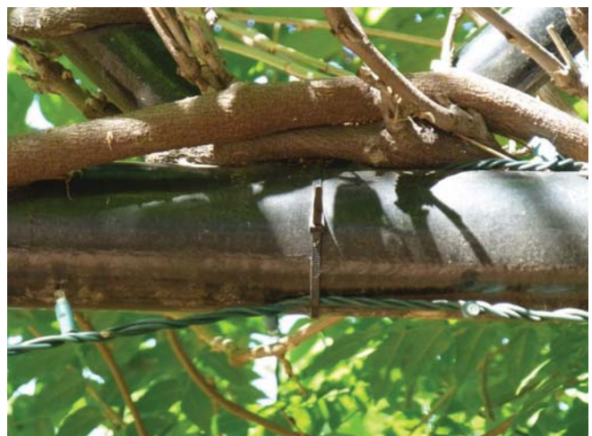
Figure 70. Zip ties have also been used to suspend strings of lights from the trellis, causing abrasion of the paint.
