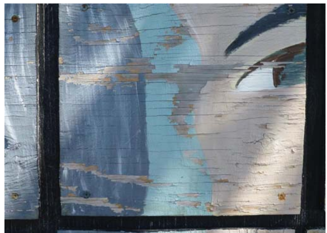
Figure 27. Typical weathering, flaking, and loss of painted finish.
