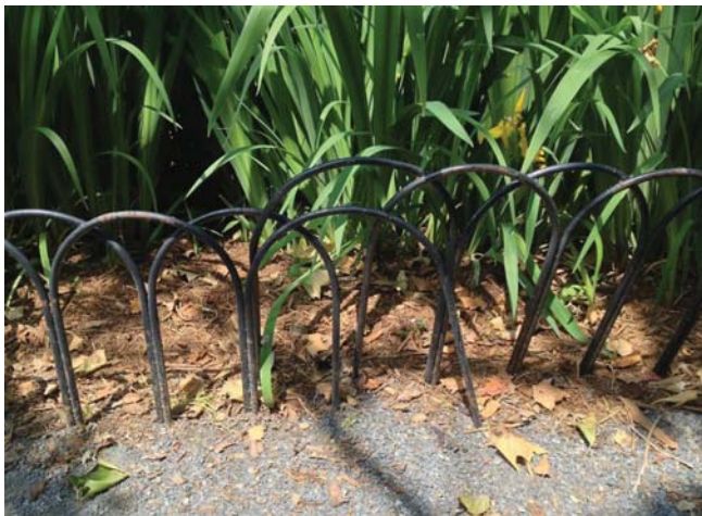
Figure 57. Some steel fencing segments have become deformed and displaced.
