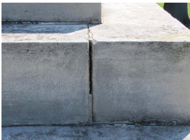
Figure 11: Typical joint exhibiting failing and lost mortar.
