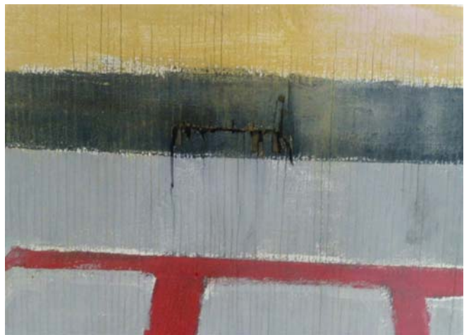
Figure 85. Example of a splintering wood surface.
