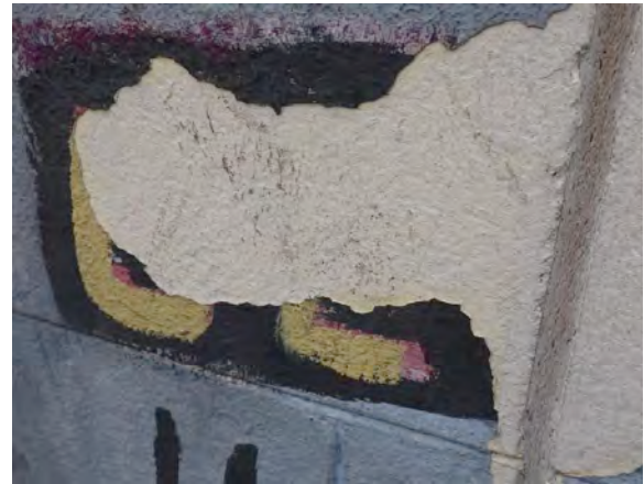
(Right) Figure 4. Flaking of the topcoat reveals the primer underneath.
