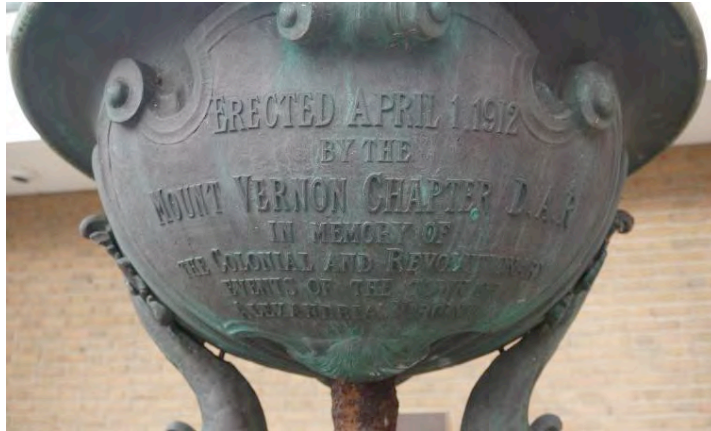
Figure 3. Corrosion on dedicatory inscription on the underside of the upper fountain basin.
