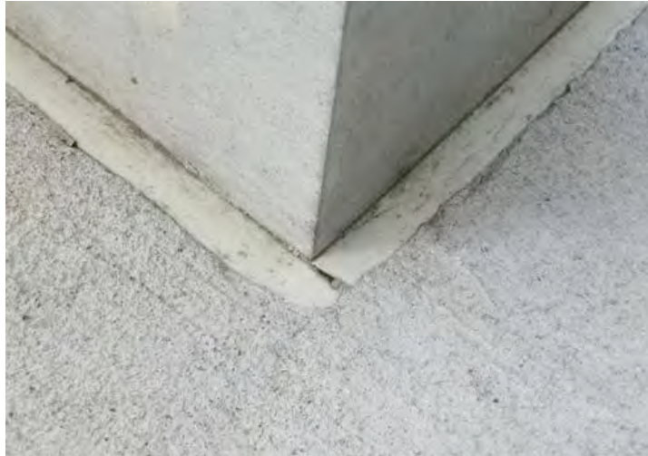
Figure 4. Detail of rigid plastic sealant embedded around the base of a pillar.
