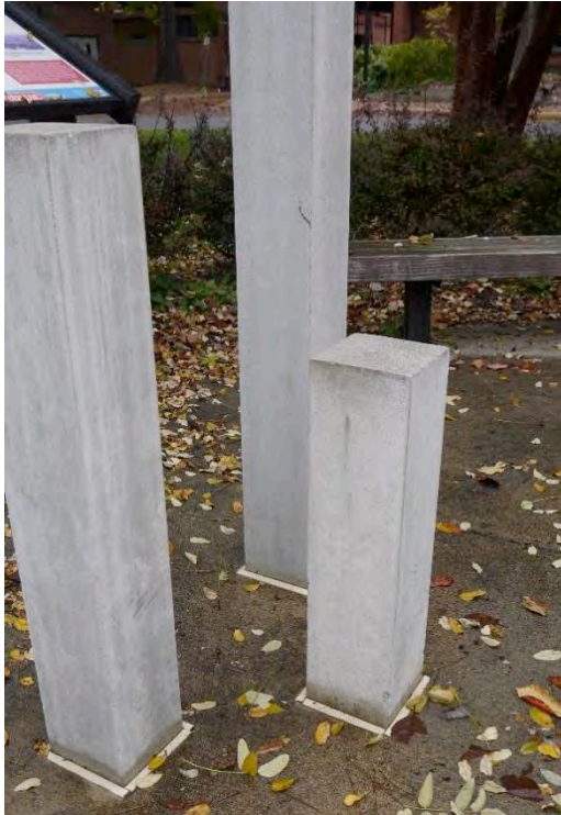
Figure 3. Detail of typical water run- off/streaking pattern down the face of the pillars
