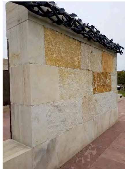
Figure 8. East wall (interior facing) with blanching and discolored patinated bronze plaques.
