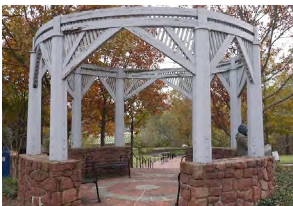
(Left) Figure 1. Part A, wooden trellis in poor condition.
