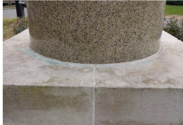
Figure 4. Detail of copper corrosion stains on the limestone base from the bronze plaque.
