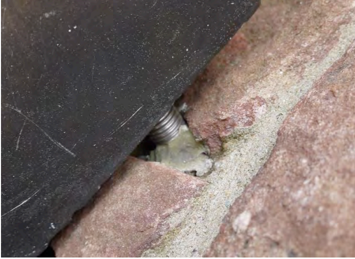
Figure 7. Detail of steel rods and epoxy securing bronze signage to brick, Part A.
