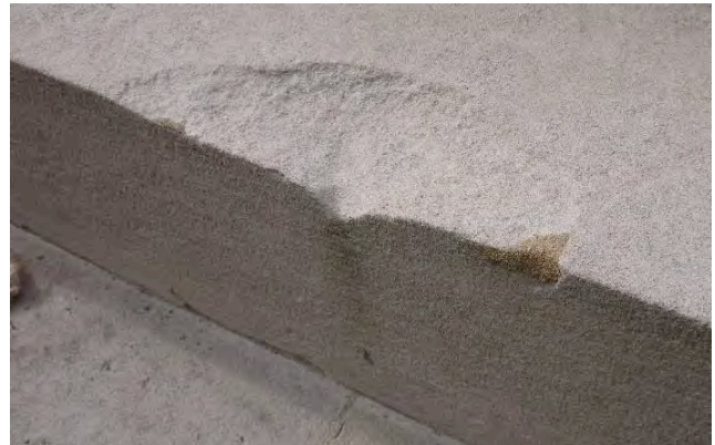
Figure 6. Limestone spall along the base.
