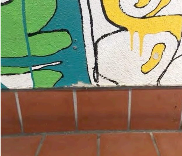
Figure 3. Detail of flaking paint along lower edge of wall.
