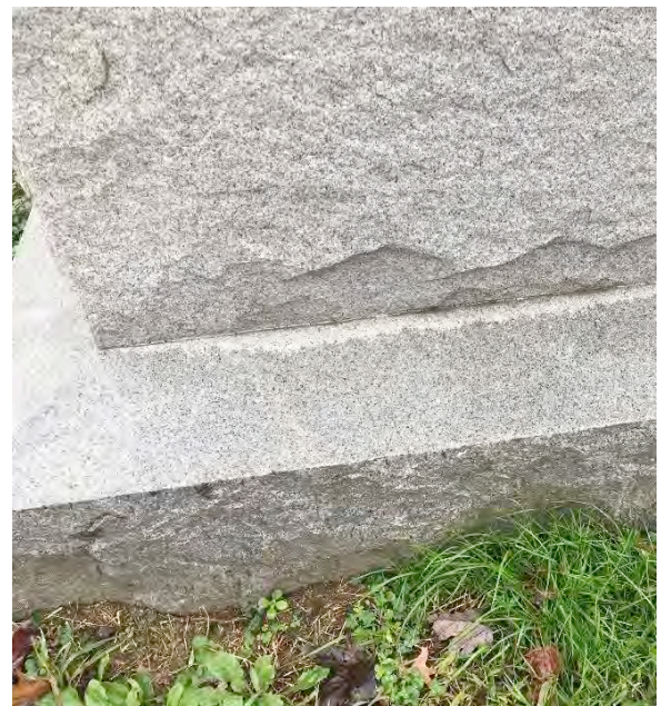
Figure 4. The lead joint between the obelisk and plinth is in excellent condition.
