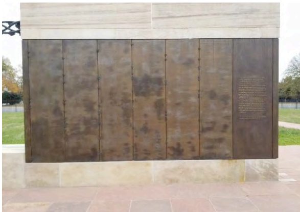
Figure 7. View of the north wall (exterior facing). Iron staining in this location is inherent to the stones.
