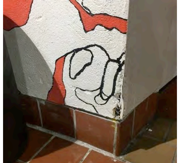
Figure 4. Large abrasion and flaking paint on bottom corner of wall.
