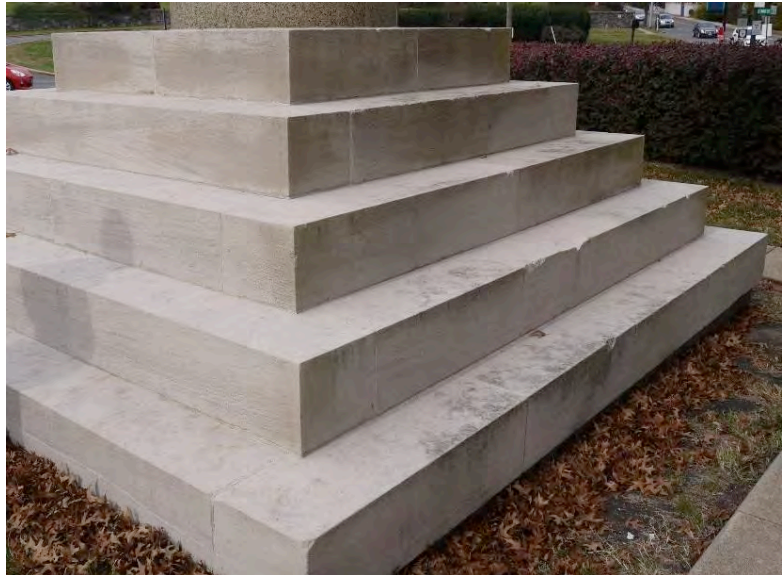
Figure 2. Detail of north elevations of the limestone steps exhibiting atmospheric spoiling and bio growth.
