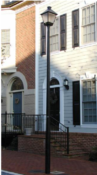
Dominion Virginia Power colonial light fixtures
