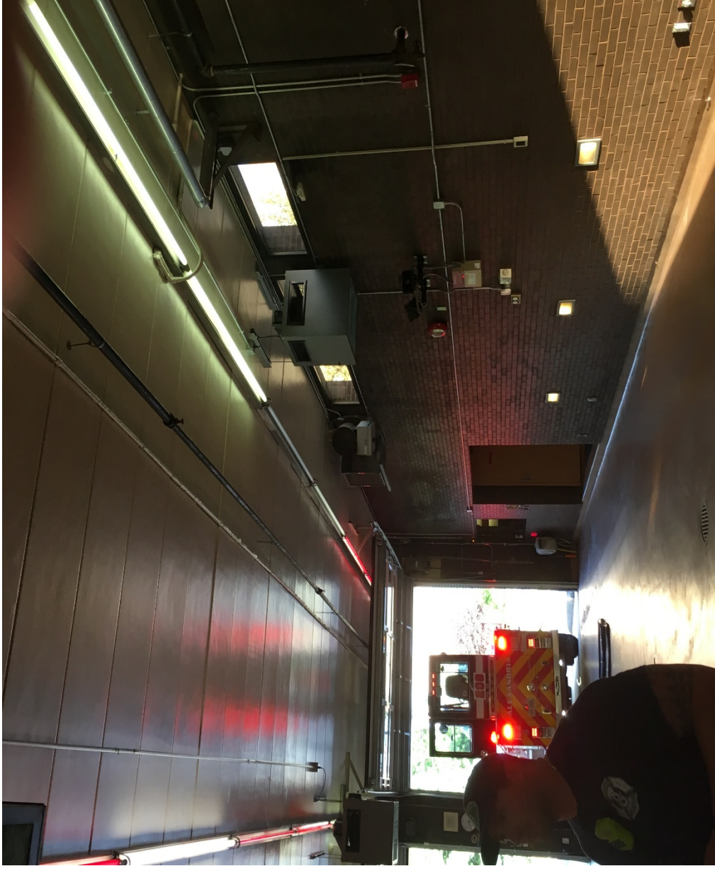
Photo # - 11. This picture is of the engine bay ceiling area where the roof is leaking.
