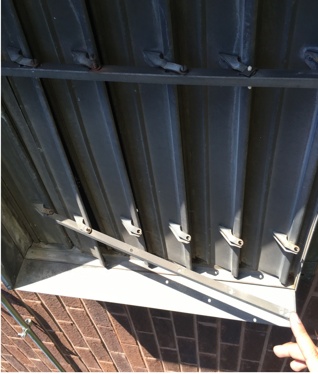
Photo # - 4. This picture is of the mechanical room exhaust fans backdraft damper which is falling apart.
