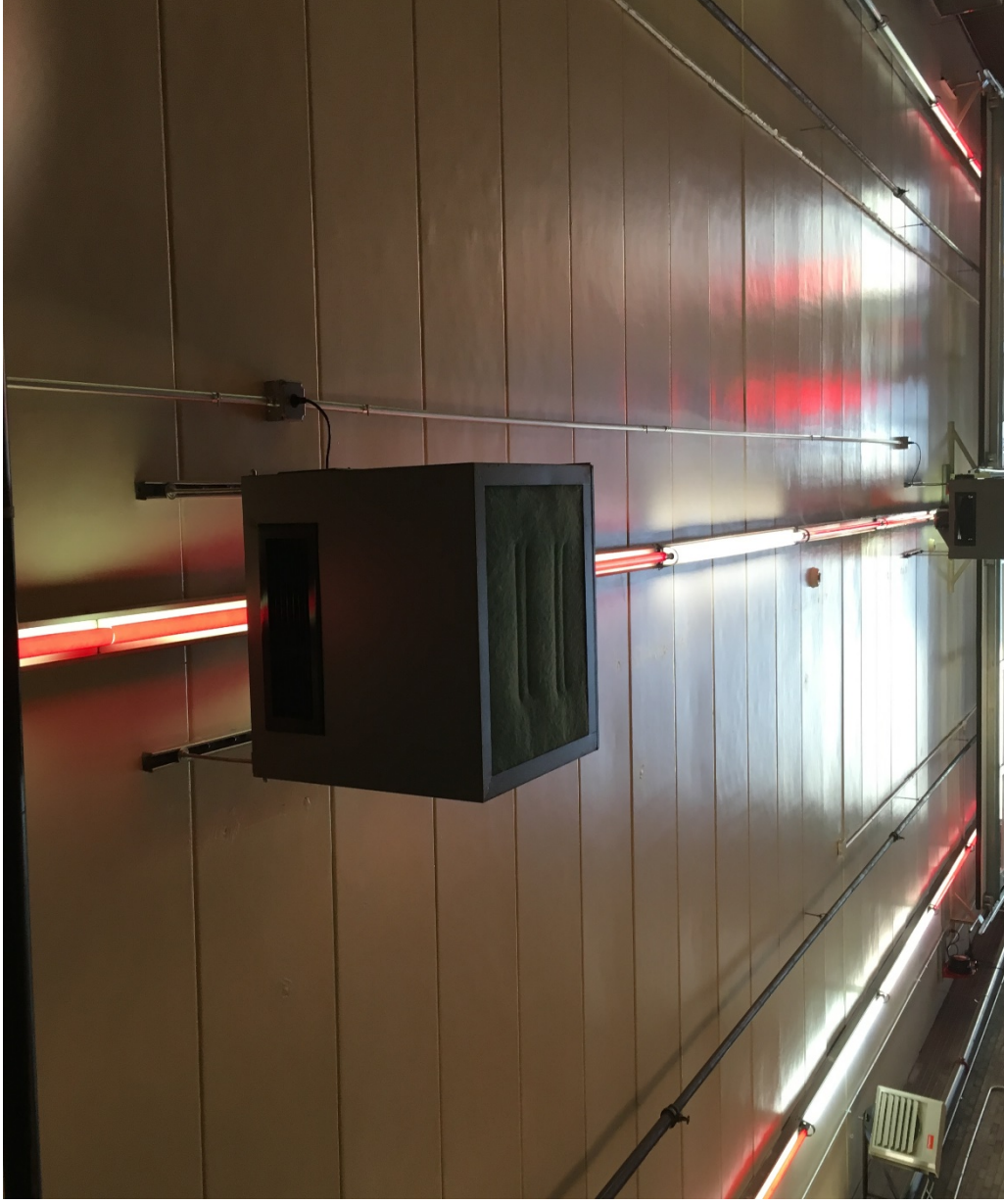
Photo # - 2. This picture is of one of the main electric unit heaters which heat the engine bay area.
