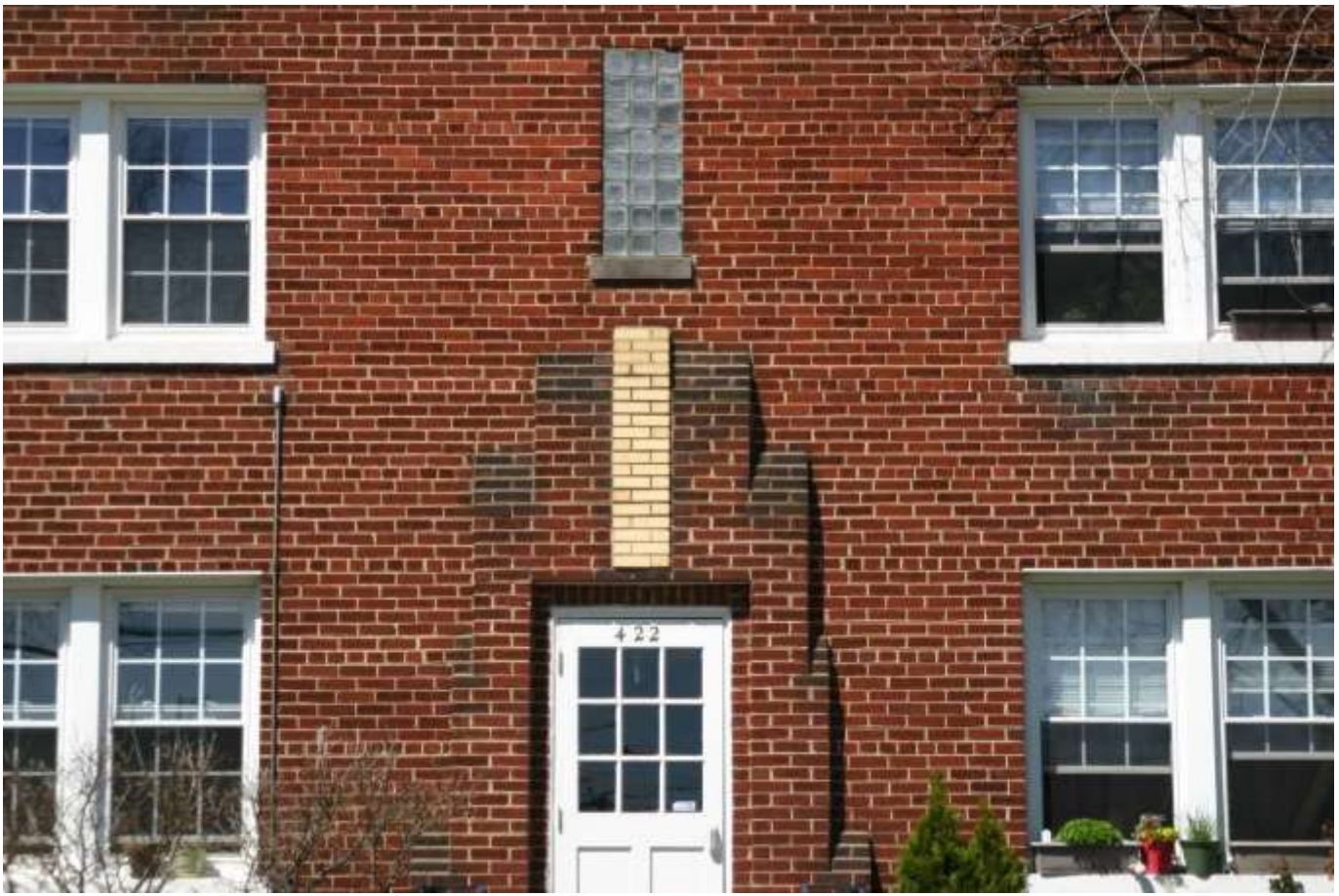
3. 422 E. Glendale Avenue. Facade (south elevation), detail: door surround and glass block window, straight angle, facing 350° N. Photograph by Gwen White 4/6/2014.
