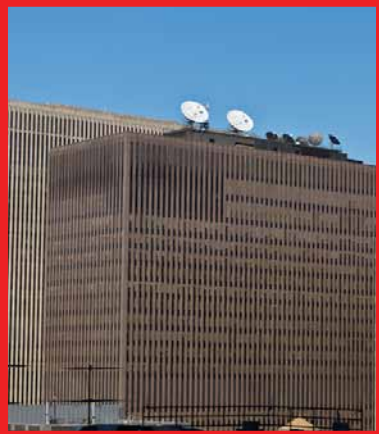
AVOID Exposed mechanical equipment, lack of tower top expression.
