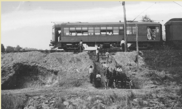
Originally a steam railroad, the line added electrical power during 1912-1916, and then switched to diesel in 1942. Here electric motor car No.43 gingerly passes over the underpass being excavated for Russell Road (just south of Glebe Road) in 1916 en route to Alexandria Junction.
