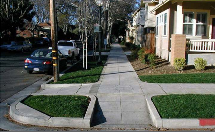
Curb ramp designed without flares. Note: detectable warning strips must be provided
