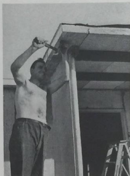
Built in an experimental housing project of the RSA at Alexandria, Va., these houses of precast concrete are now reaching completion, from plans by Kastner and Hibben, architects. Slabs are used for floors, walls and roof, with a board type insulation above the roof slabs. Houses of stabilized earth block and of rammed earth are also part of the project.
