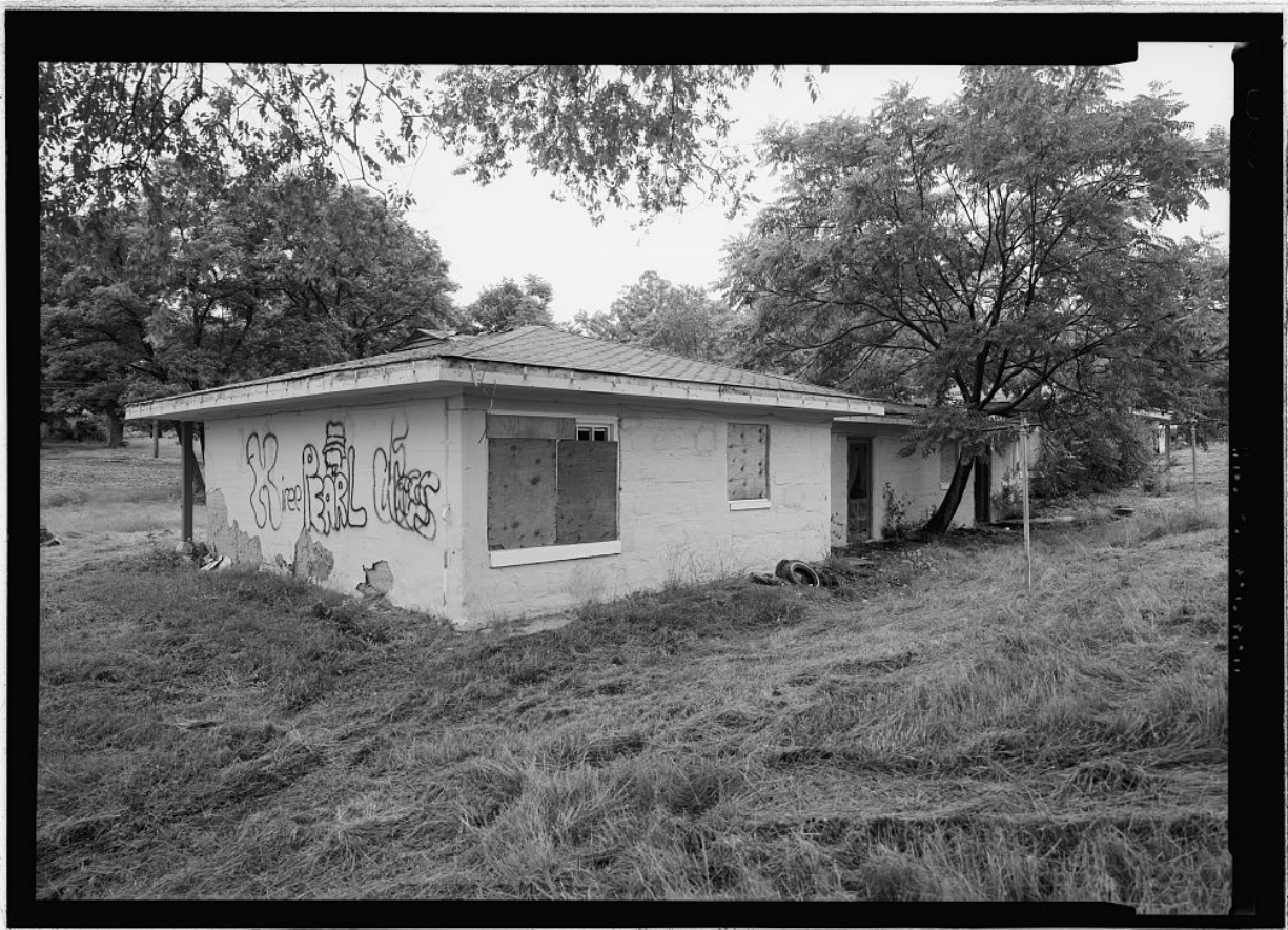
Figure 23: Perspective View of Alexandria Housing Authority, Cameron Valley Housing, Alexandria, Virginia (Lowe 1988)
