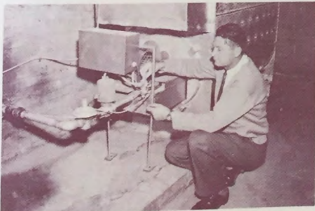
Oil Burner Installation Inspection
