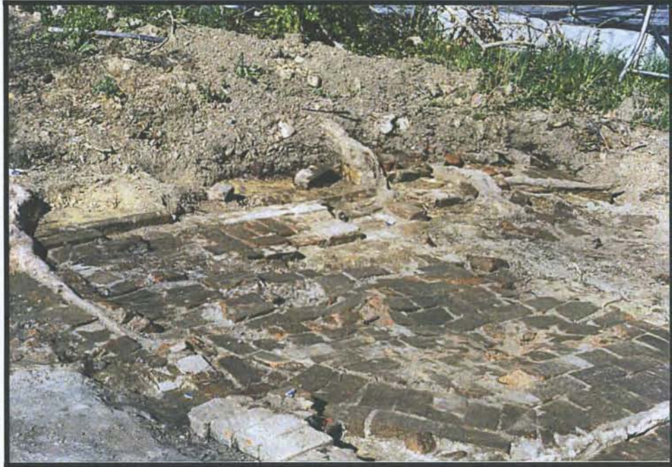
Figure 69. Overview of greenhouse structure, showing laid brick floor, surrounding foundation walls (orientation northeast)
