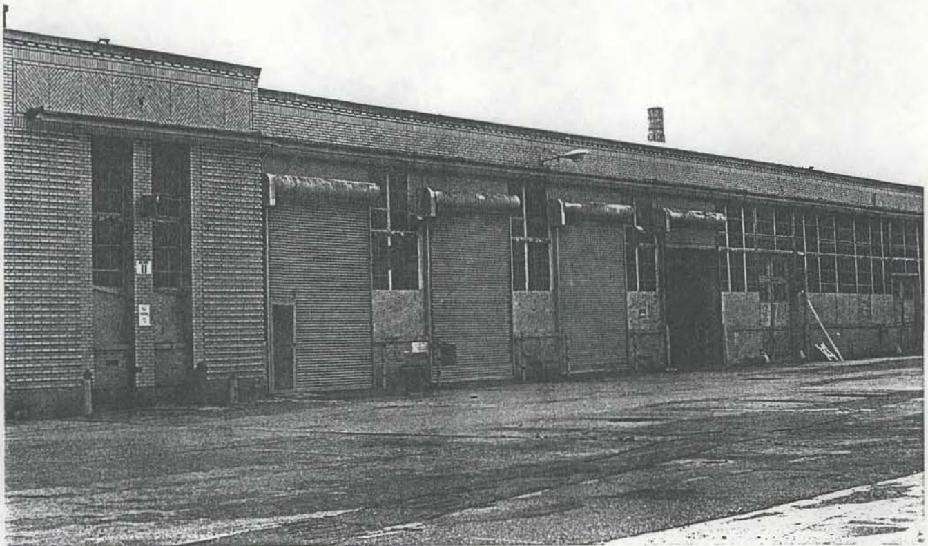
Photograph of a portion of the south elevation of the 1932 Old Ford Plant building (#11).
