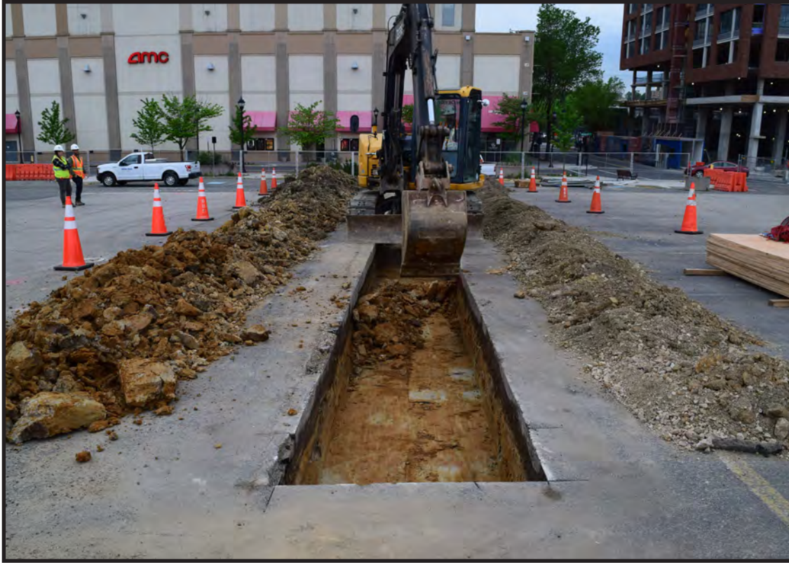
Figure 2.11 Photograph showing backhoe removing soil in shallow lifts (levels), Trench 3, view south
