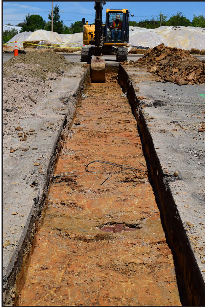
Figure 3.6 Trench 2: Photograph showing utilities and subsoil exposed in trench, plan view facing north (38 cm below surface)
