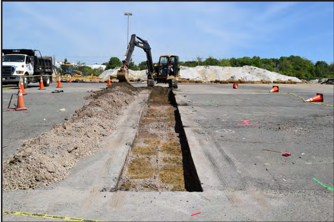
Figure 2.10 Photograph showing backhoe stockpiling gravel base from parking lot at Trench 2, view north
