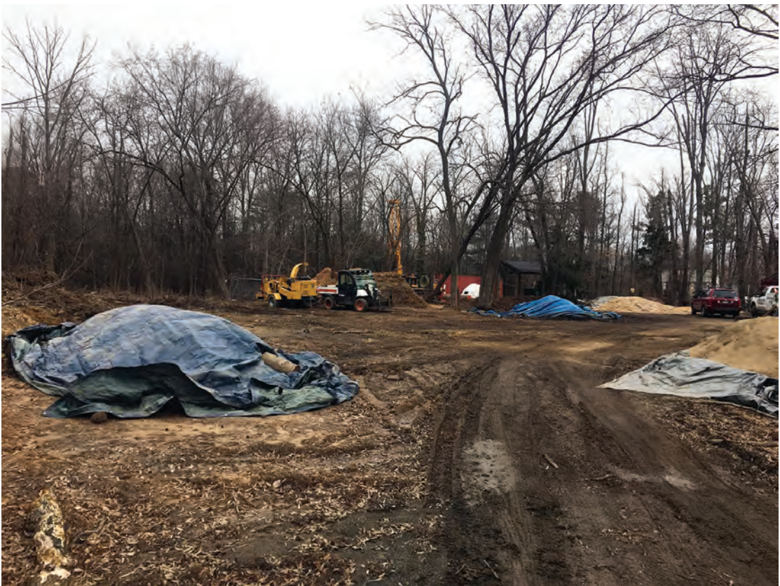
Figure 21. Maintenance yard showing disturbance, facing north.
