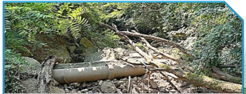
Existing condition of at-risk sanitary sewer line
