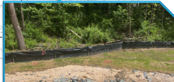
Super Silt Fence
