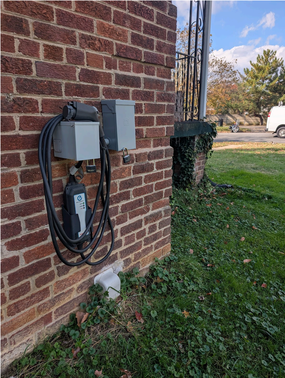
Exhibit 3 - photograph of existing permitted and installed electrical vehicle charging port
