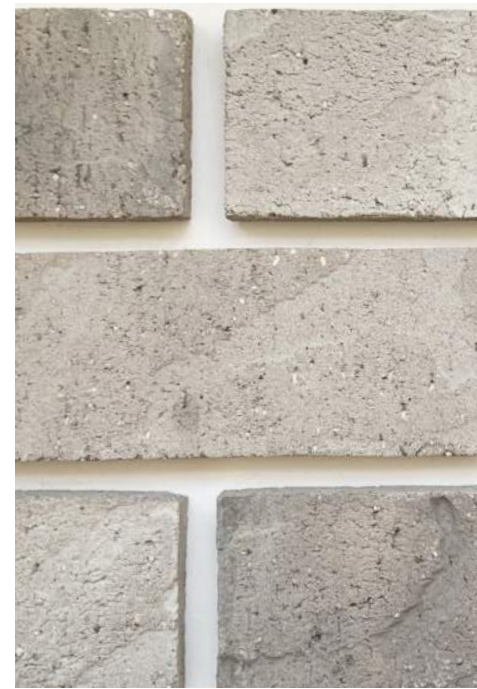
WEATHERED BRICK 1 SAMPLE
