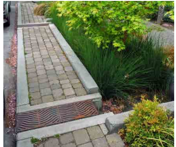
Stormwater management BMP.
