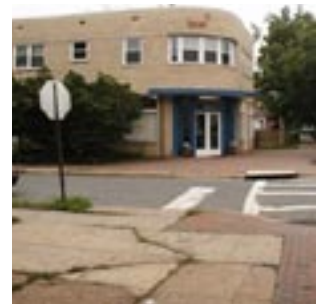
Poor quality pavers
