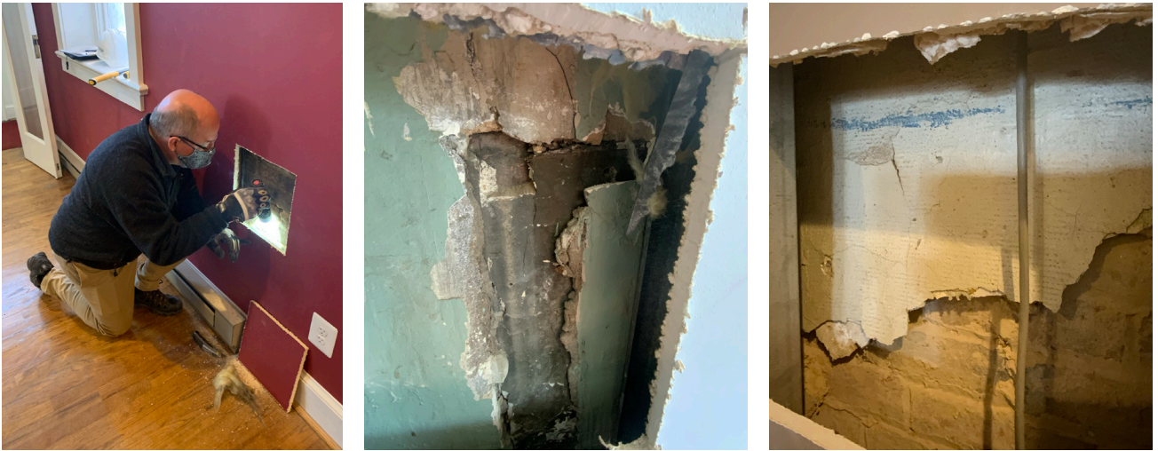
Figure 02: Images showing process of investigating behind existing modern drywall finishes to uncover evidence of historic 3-coat plaster.
