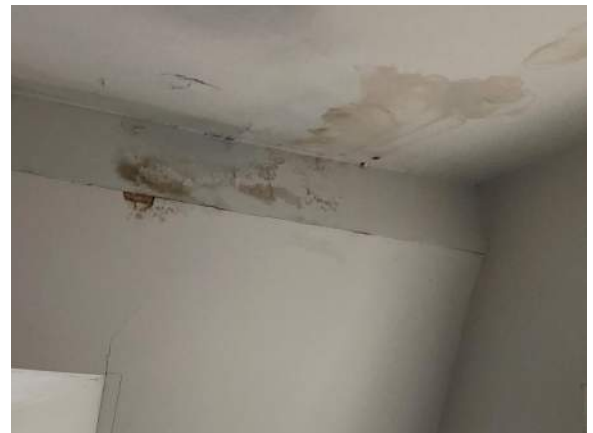
Figure 2E-8: Water damage at ceiling in Office 403 on fourth floor/ mezzanine.
