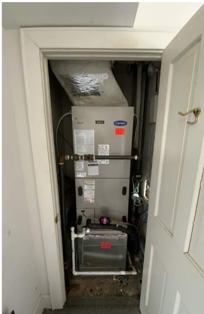
Mechanical Closet 403A
