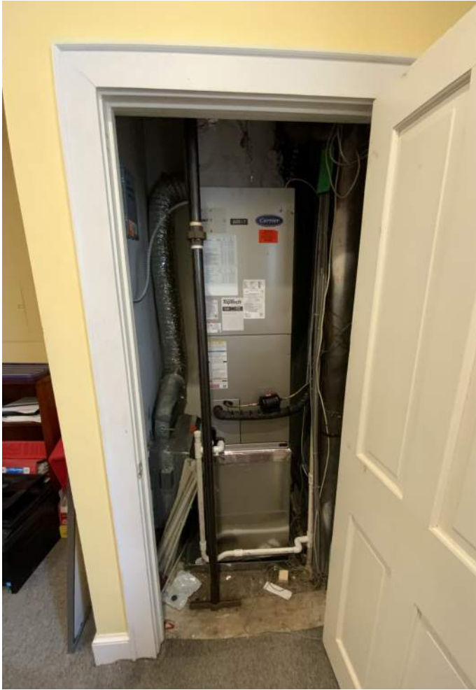
Mechanical Closet 304A
