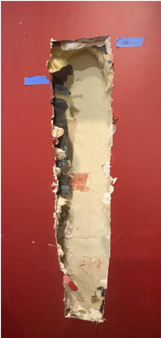
Figure PR12-1: Opening cut in existing drywall along the east wall of Office 304 at Chimney #2.
