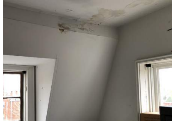
Figure 2D-8: Staining and bubbling of drywall finish in northeast corner of mansard roof within Office 403 in the South Block.
