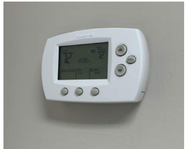
Figure 2D-18: Thermostat providing temperature control to air conditioning unit
