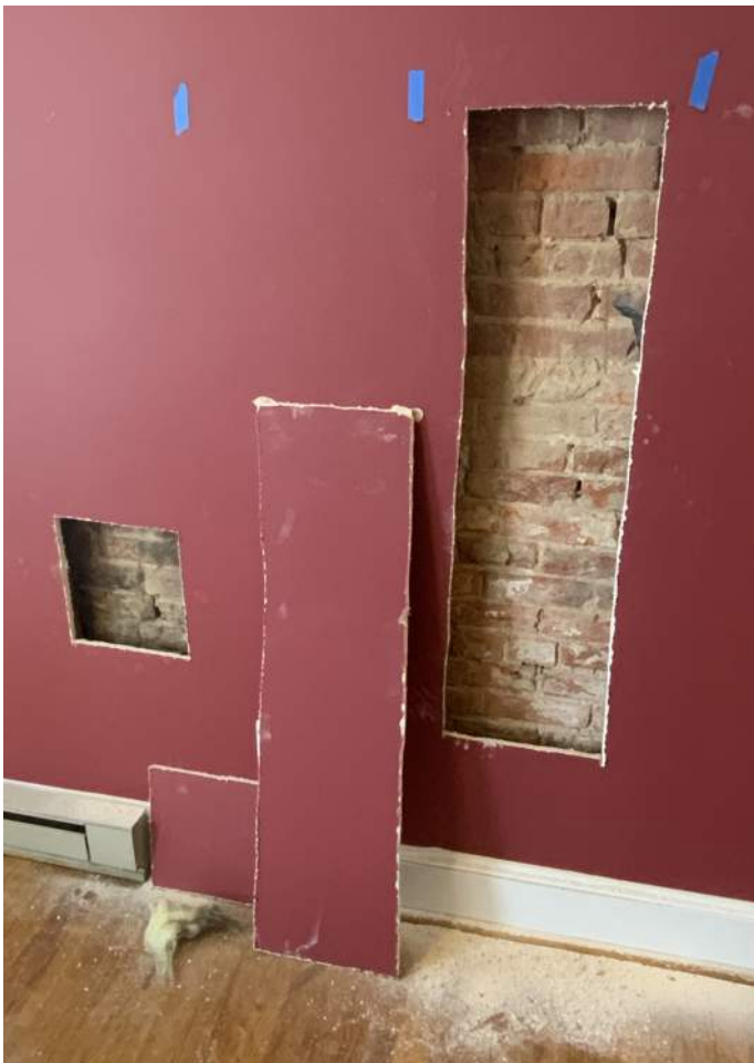
Figure PR1-1: Two (2) openings cut in existing drywall finish along west wall of Corridor 102.
