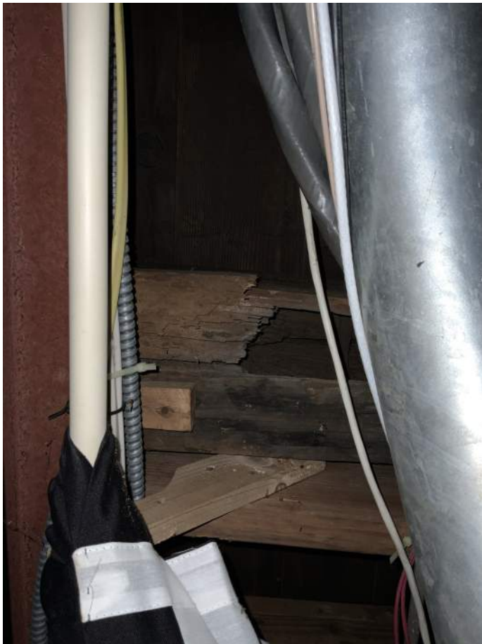
Figure PR19-1: Evidence of significant wood rot and deterioration at the bearing end of historic floor joists.
