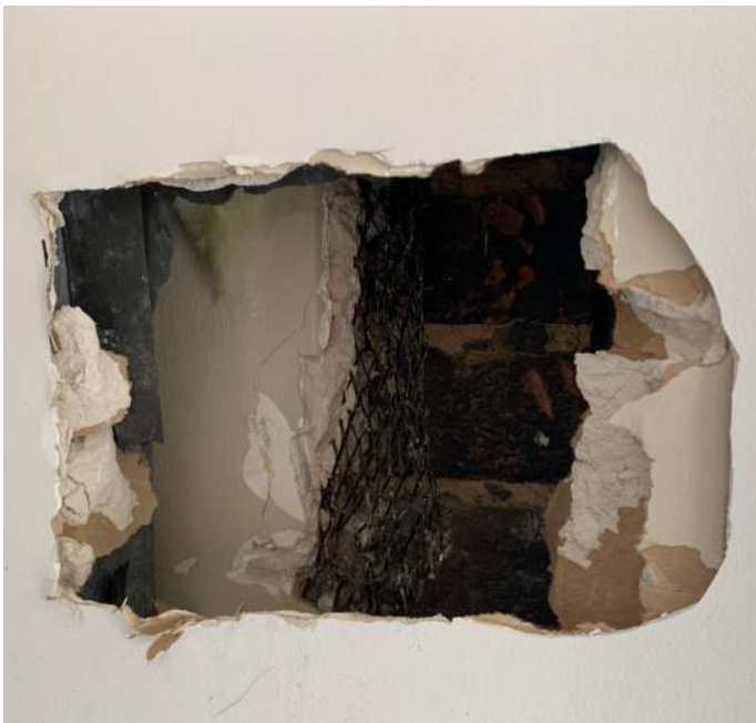
Figure PR18-1: Opening cut in existing drywall along the east wall of Office 403 at Chimney #2.
