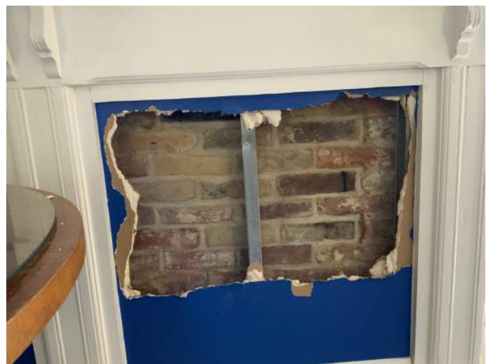
Figure PR17-4: Opening cut in existing drywall along the east wall of Office 402 at Chimney #1.
