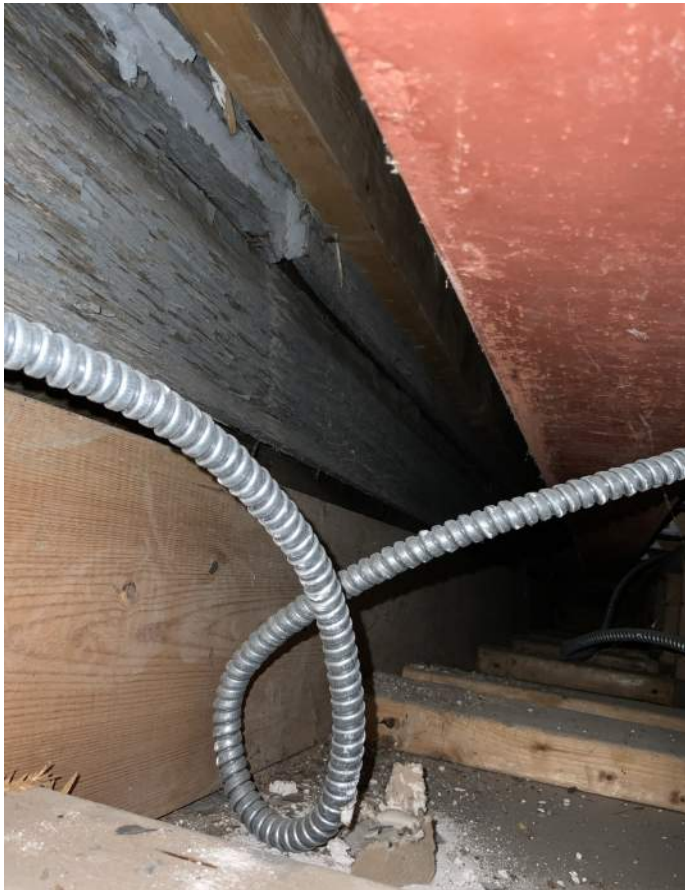
Figure PR9-1: View within probe #9 looking north locating the steel beam installed during the 1985 Addition and the remaining wood siding installed in 1937 per Permit #2415.
