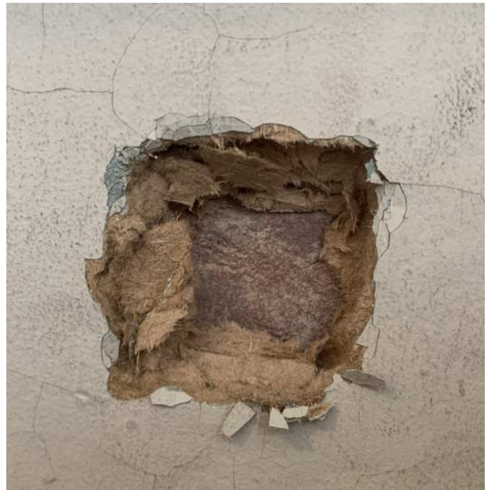
Figure PR2-2: Detail photo of wood fiber insulating board installed along historic brick masonry wall.
