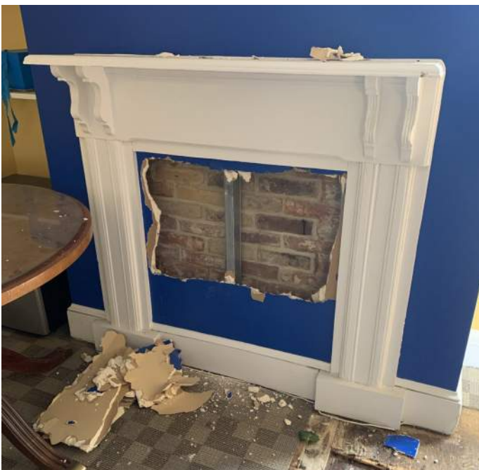
Figure PR17-3: Opening cut in existing drywall along the east wall of Office 402 at Chimney #1.
