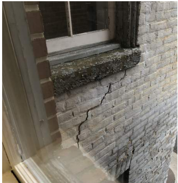
Figure 2D-12: Large crack at east return of North Elevation, located under masonry opening 219 of the North Block.
