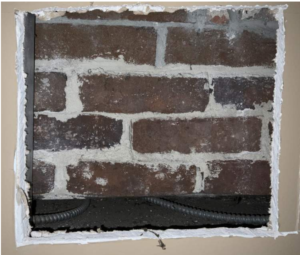
Figure PR14-1: Opening cut in existing drywall along the south wall of Corridor 305A above masonry opening 308.
