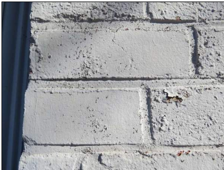
Figure 13: Detail of mortar at infill around windows. Note the smooth brick and the flat joint profile.
