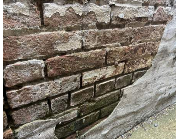
Figure 2E-1: Missing mortar in west alley near grade.
