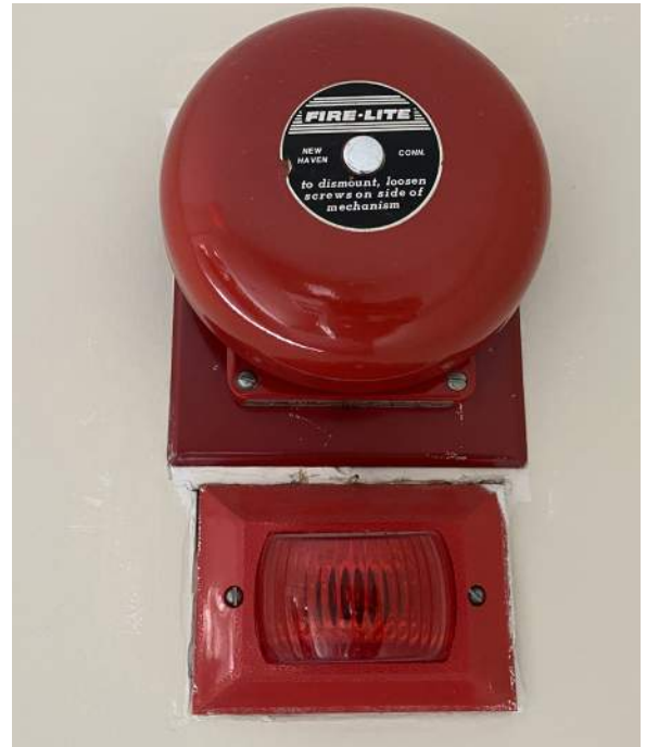
Figure 2D-36: Fire alarm audible bells and non-ADA compliant flashers.
