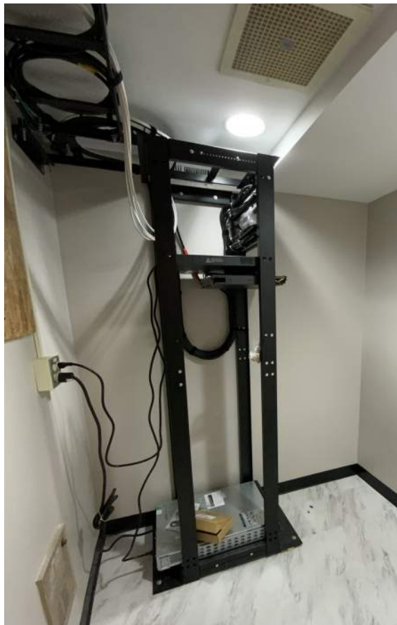
Figure 2D-28: Existing IT rack on second floor.
