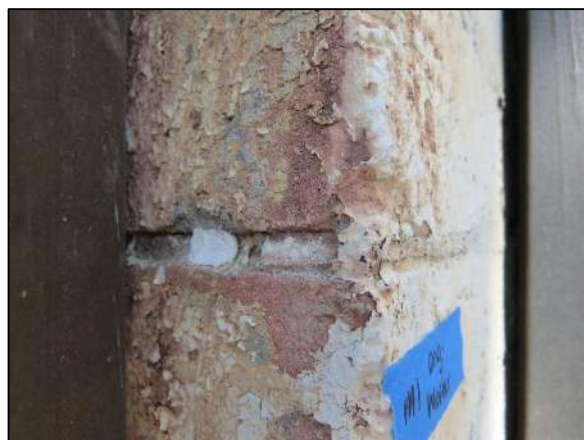
Figure 30: Location of Sample M-1 behind the downspout.
