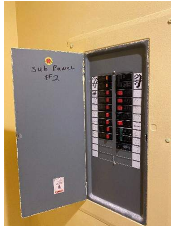
Figure 2D-26: Existing sub-panel #2
