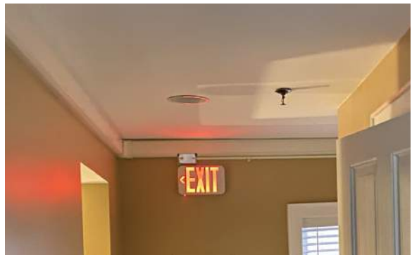
Figure 2D-35: Sprinkler head located too far from wall for coverage.
