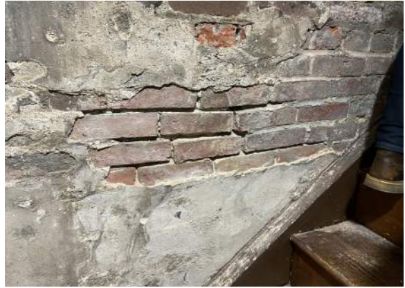
Figure 2D-11: Failing parge coat observed at east wall of Basement at Stair 1, located along west foundation wall.
