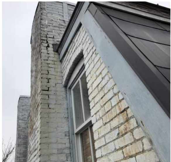
Figure 2D-14: Upper portion of east elevation of South Block; Note the poor condition of Chimney #2 and the prior repairs.
