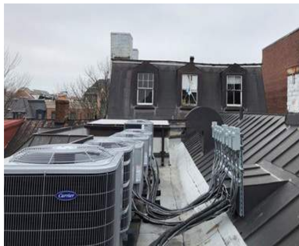
Figure 2C-10: Roofs viewed from the south end of the structure looking north. Note the flat roof of the 1980s addition, gable roof of the northwest portion, and mansard roof of the south portion.
