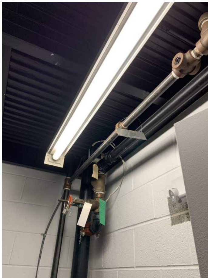
Stair 3, Standpipe in corner of egress stair
