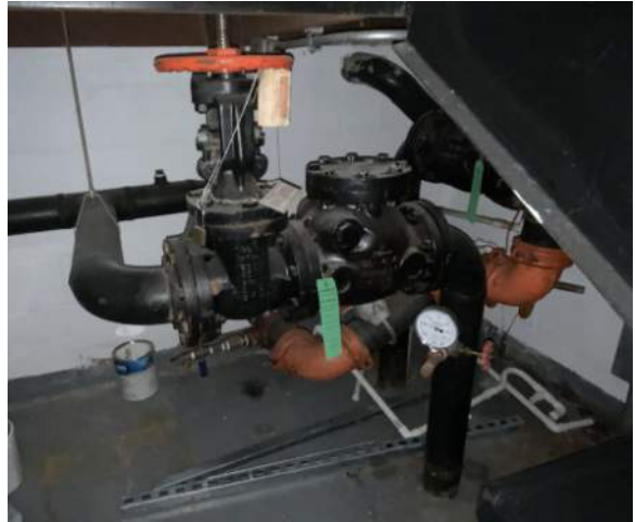
Figure 2D-31: Incoming fire service partially obstructed by storage.
