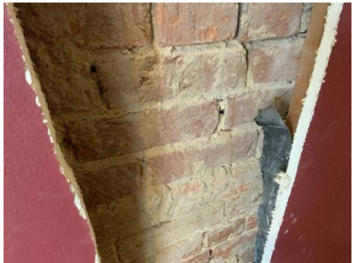
Figure PR1-2: One of two openings cut in existing drywall finish along west wall of Corridor 102. Existing wood stud framing found installed along historic brick masonry. A few cut nails were found within the mortar joints.
