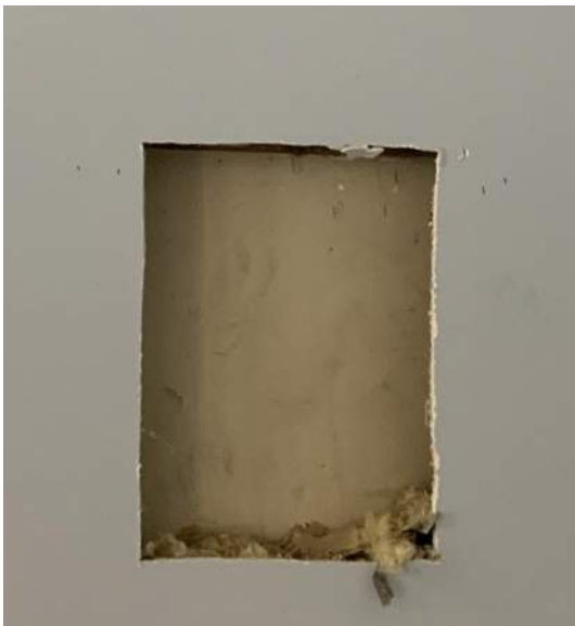
Figure PR6-1: Upper and lower openings cut in existing drywall along west elevation of Conference Room 201.
