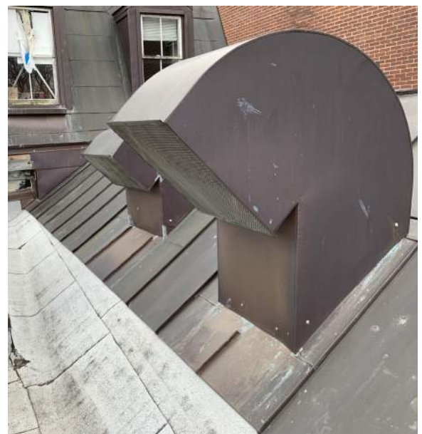
Figure 2D-20 Air intake and toilet exhaust
