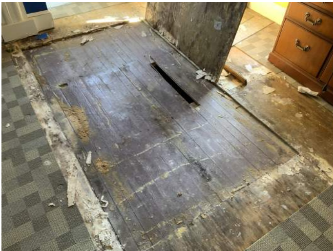
Figure PR16-1: Historic wood flooring uncovered from beneath a plywood subfloor and carpet tile.
