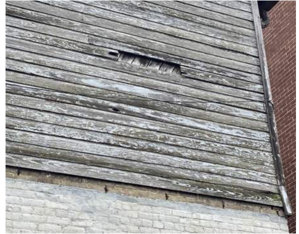
Figure 2E-6: Sheathing and siding damage at historic North Block (Period 4B).
