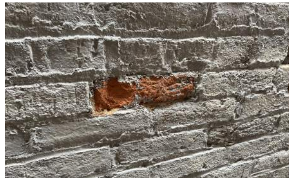
Figure 2E-3: Spall in brick masonry unit.
