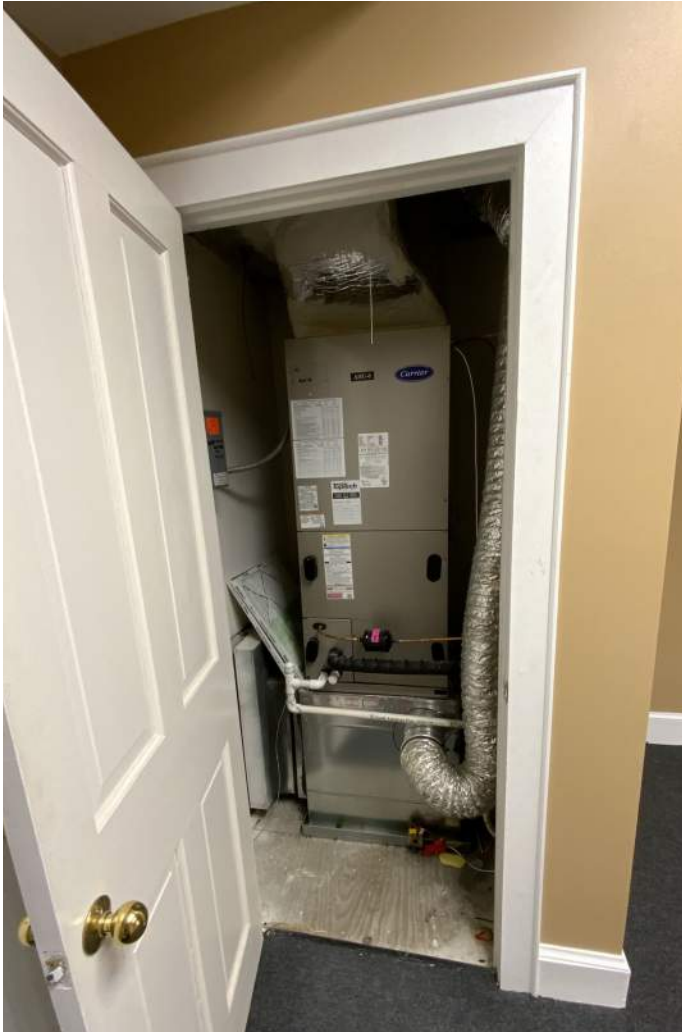
Mechanical Closet 310A
