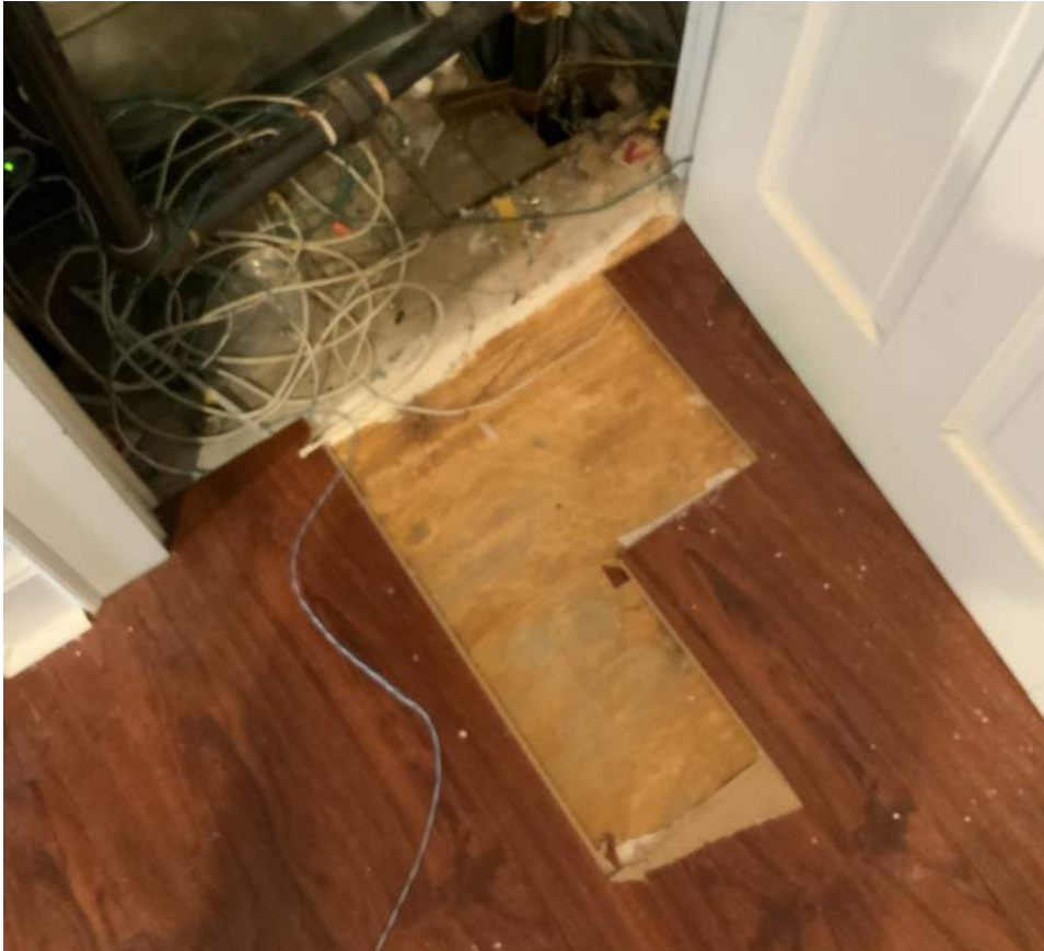
Figure PR8-1: Plywood subfloor uncovered beneath the existing laminate floor. The wood flooring in the adjacent mechanical closet may be original.
