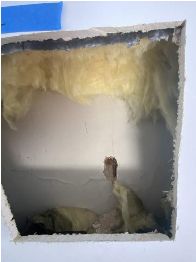
Figure PR10-1: Opening cut in existing drywall along the south wall of Office 302.
