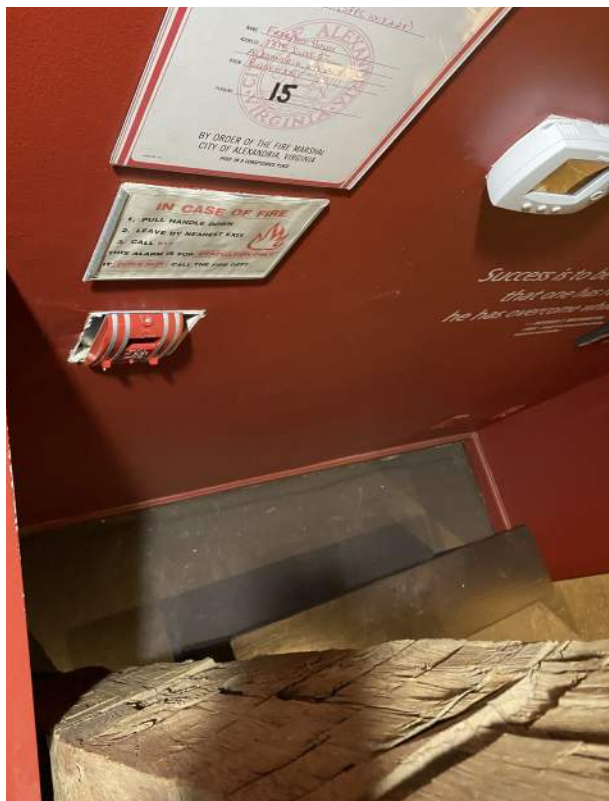
Figure 2D-38: Fire alarm manual pull station obstructed by exhibit at basement level.
