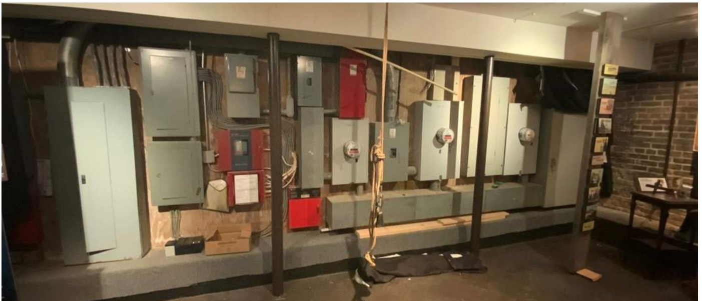
Figure 2D-27: Electrical Service Entrance Equipment - Basement Level
