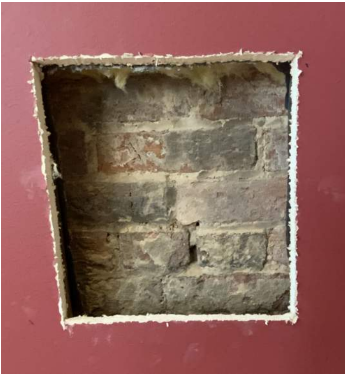
Figure PR1-3: One of two openings cut in existing drywall finish along west wall of Corridor 102.
