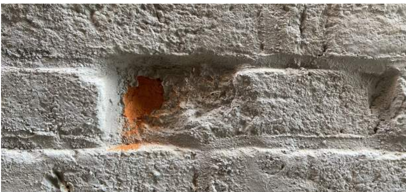
Figure 2D-13: Spalled brick face at west elevation.
