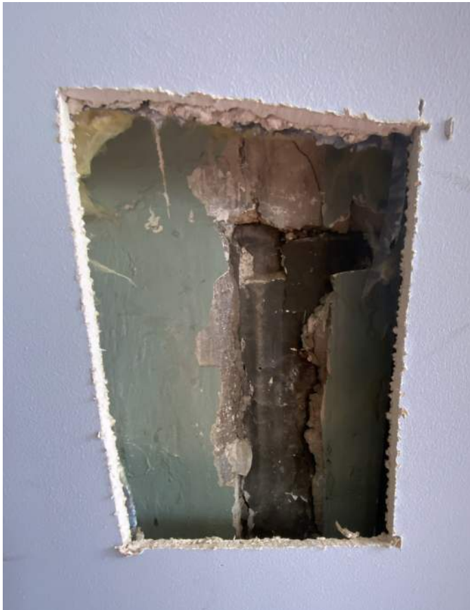
Figure PR5-1: Opening cut in existing drywall along east elevation of Conference Room 201 at the face of Chimney #1.
