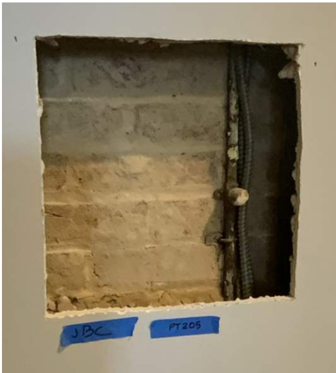
Figure PR7-1: Opening cut in existing drywall along north elevation of Office 203.
