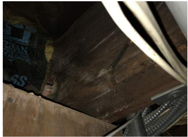
Figure 2C-4: Joist end visible from basement. Note the poor condition of the joists near the end.
