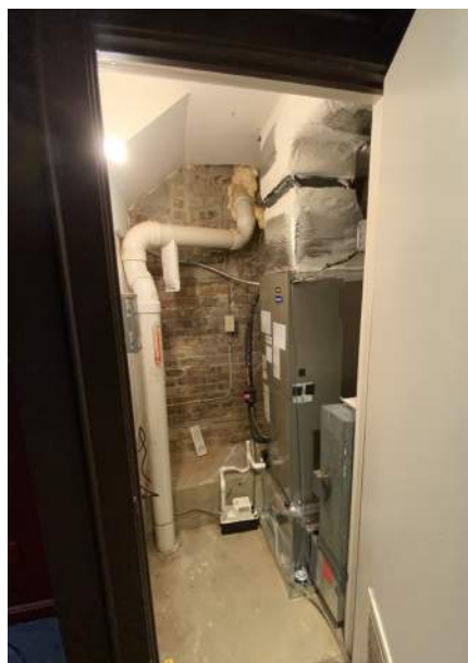
Figure 2D-19: AHU-1 with condensate return pump located in basement mechanical closet
