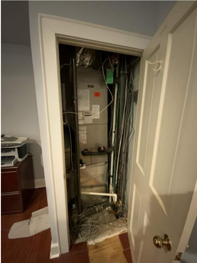
Mechanical Closet 203A
