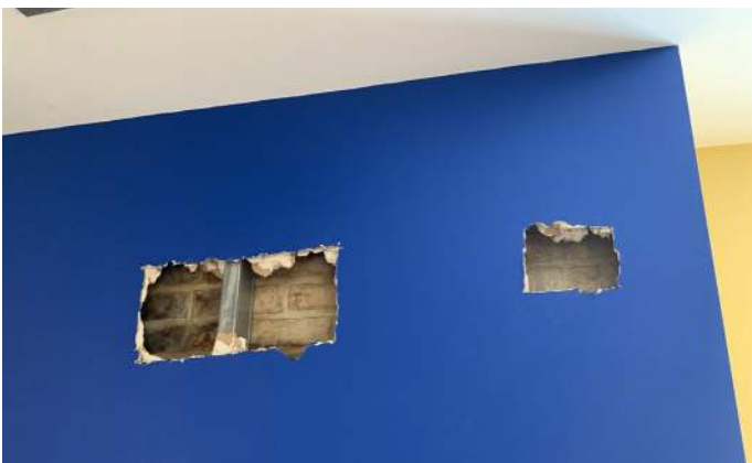
Figure PR17-1: Opening cuts in existing drywall along the east wall of Office 402 at Chimney #1.
