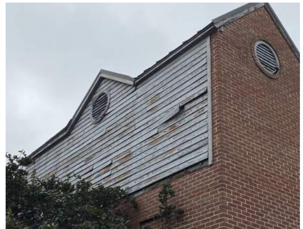
Figure 2E-7: Sheathing and siding damage at 1985 Addition (Period 5).
