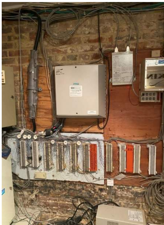
Figure 2D-29: Basement level patch panels.
