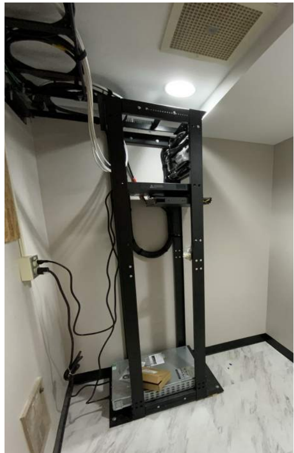
Figure 2D-21: Former restroom converted into Server Room.
