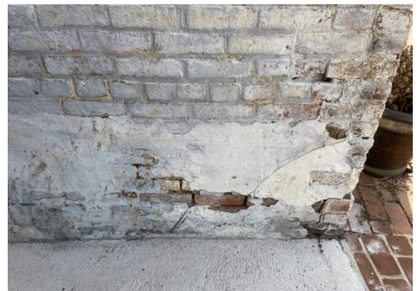
Figure 2D-10: Failed parge coat and mortar loss near grade at southwest corner of South Block
