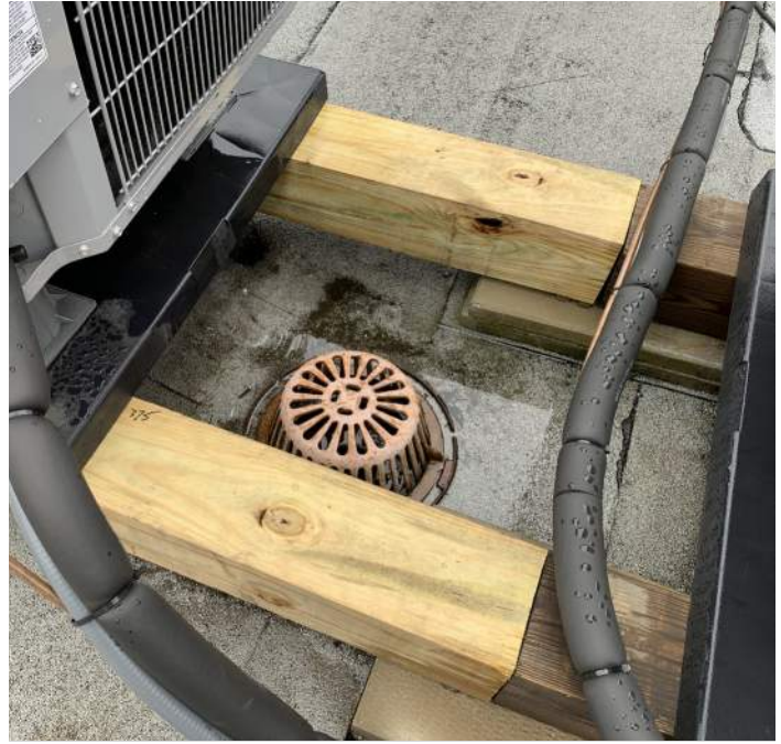
Figure 2D-25: Existing roof drain.
