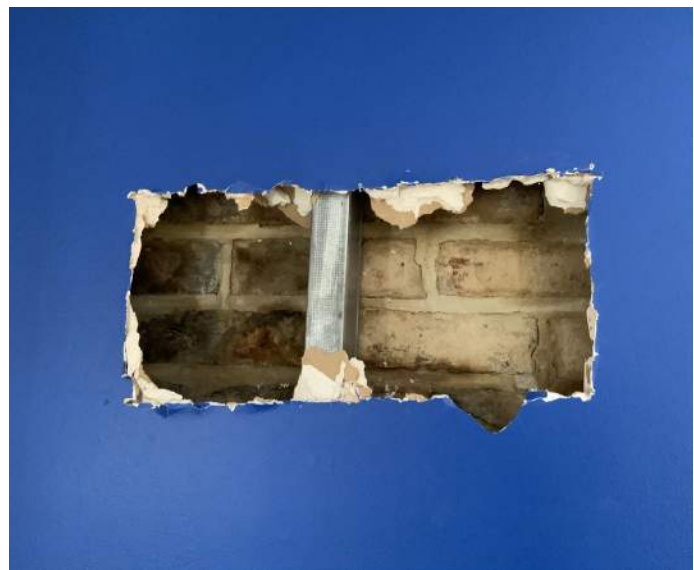
Figure PR17-2: Opening cut in existing drywall along the east wall of Office 402 at Chimney #1.
