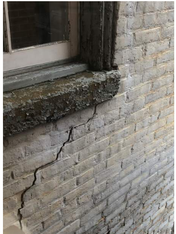
Figure 2E-2: Crack in brick masonry near rear entrance to building.
