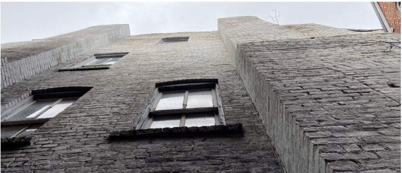
Figure 2E-5: Chimney #1 and Chimney #2 deformation at east elevation.
