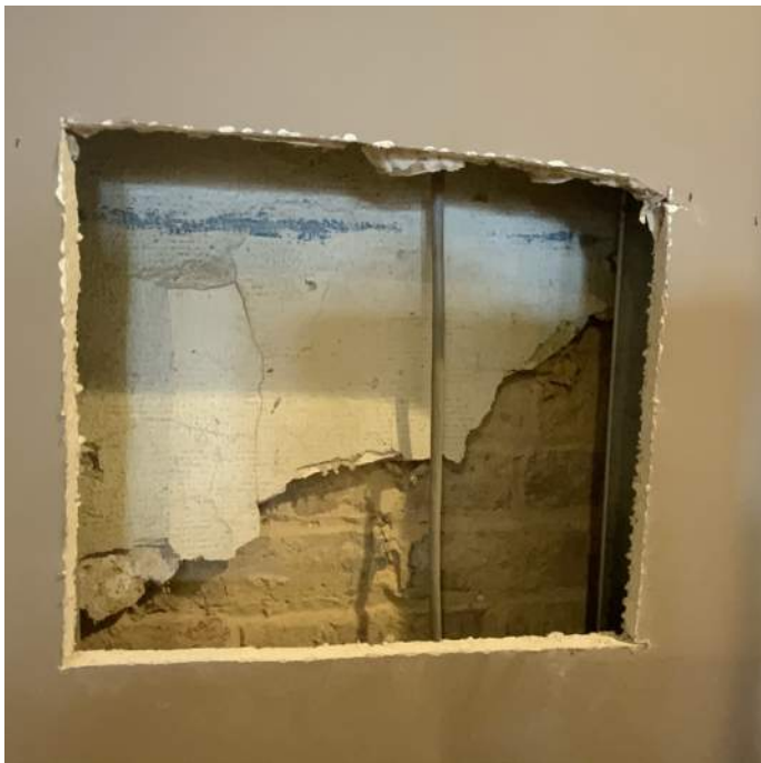
Figure PR3-1: Opening cut in existing drywall along north wall of Museum 104 just west of masonry opening 105.
