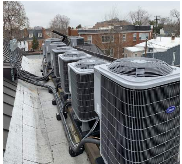
Figure 2D-17: Roof-mounted outdoor condensing units.
