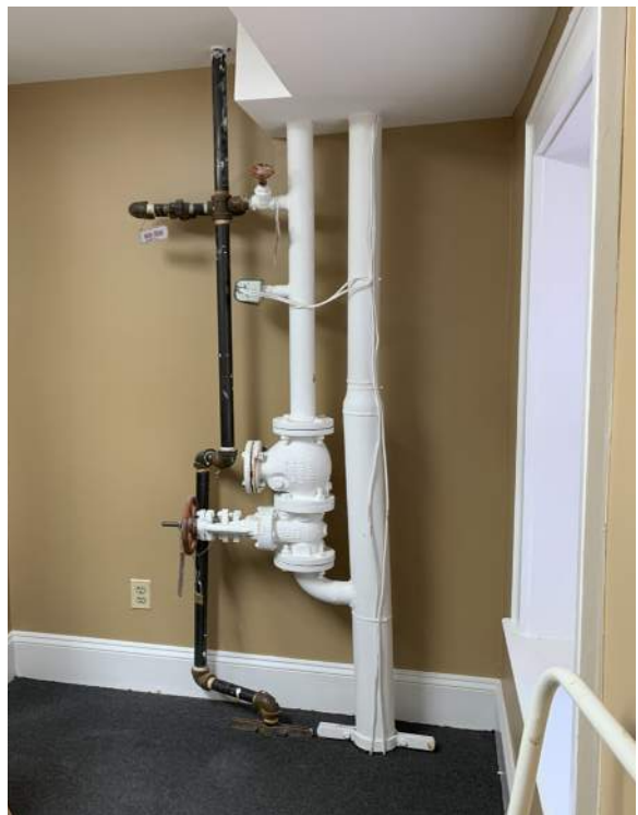
Figure 2D-32: 2-1/2" sprinkler riser with associated riser OS&Y gate valve and check valve located in the North Block.
