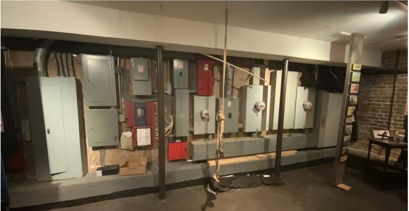
Figure 2E-9: Existing south wall of basement in South Block where the electrical service, panelboards, and other fire alarm and security devices are located.
