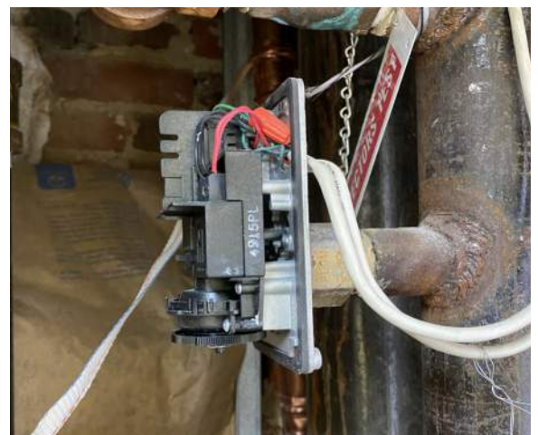
Figure 2D-39: Cover plate missing on water flow switch.
