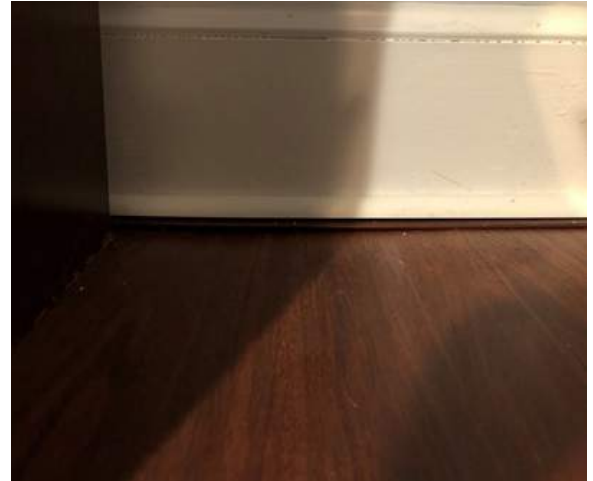
Figure 2D-5: Gap evident in baseboard trim at second floor office, opposite the corridor wall from Stair 1.
