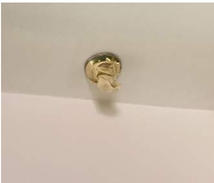
Figure 2D-33: Sprinkler head covered by masking tape.
