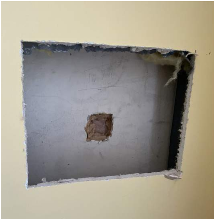
Figure PR2-1: Opening cut in existing drywall along east wall of Reception 103 just south of Chimney #1.
