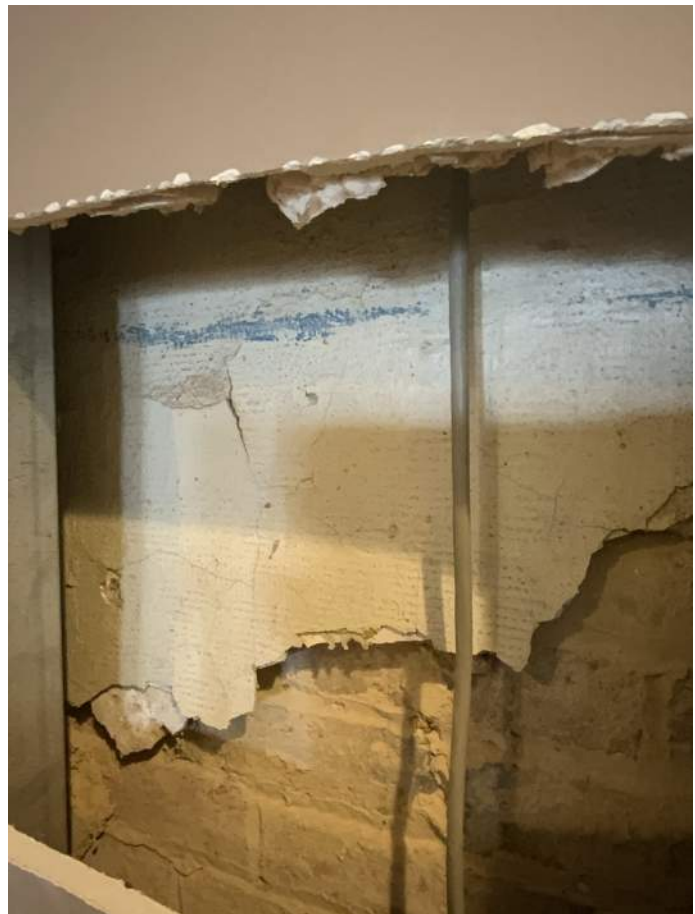
Figure PR3-2: Detail of historic 3-coat plaster found behind modern drywall finish.
