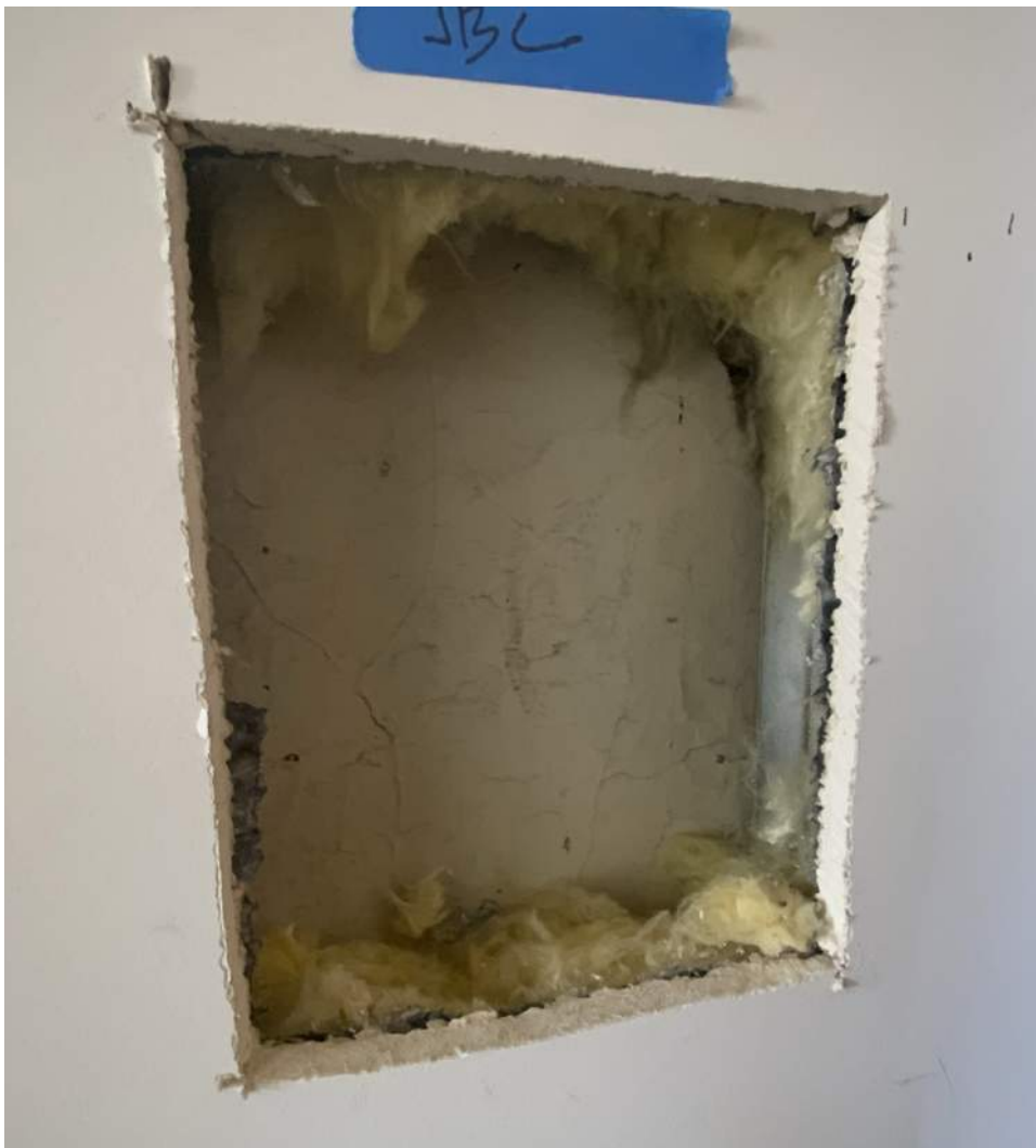
Figure PR11-1: Opening cut in existing drywall along the west wall of Corridor 303.
