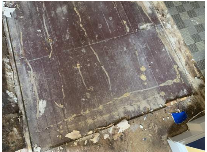
Figure PR16-2: Evidence of prior attic access through hinged panel in the floor.
