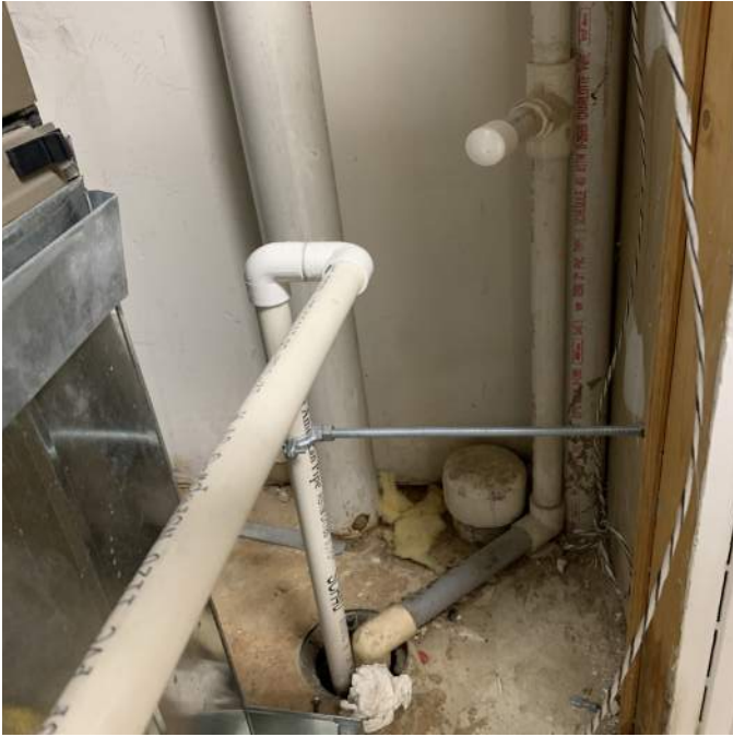
Figure 2D-24: Sanitary drain pipe and floor drain in mechanical closet
