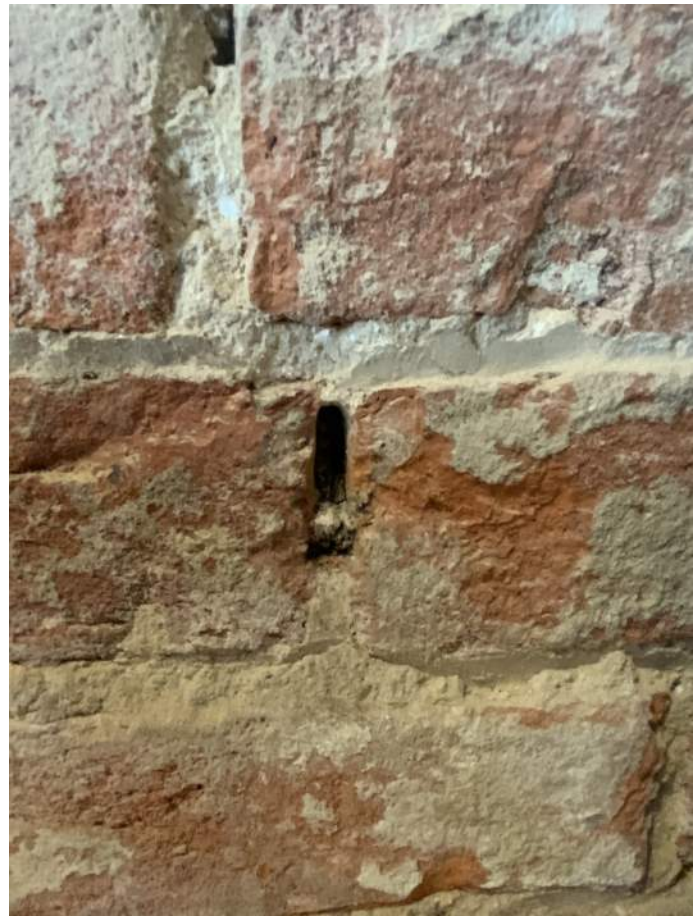
Figure PR1-4: Fragment of wood blocking found within the mortar joint.
