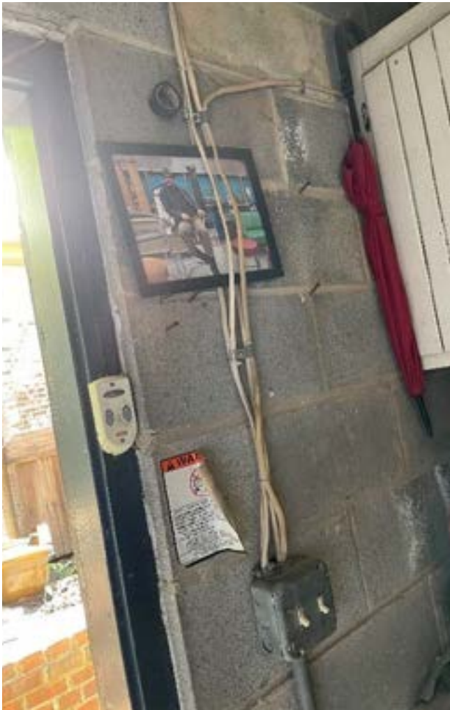
Figure 20ab. - Incoming Branch Circuits to equipment in the Garage.
