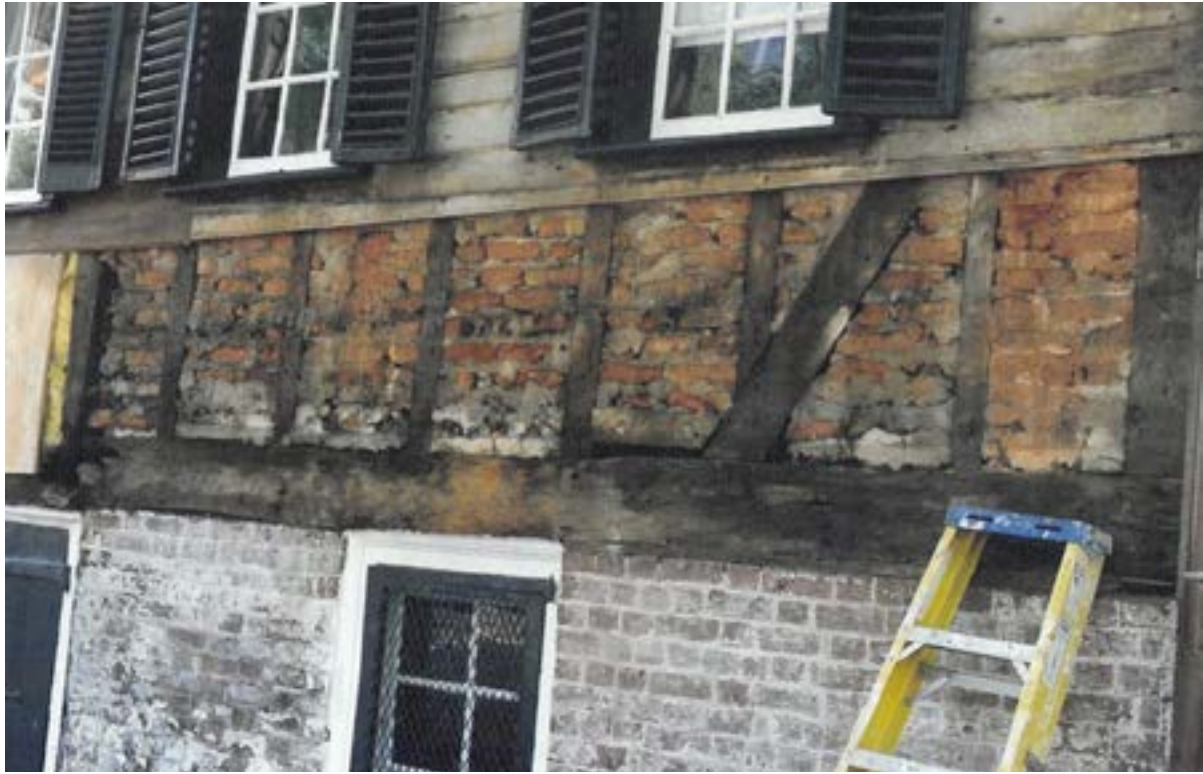
Figure 8e. - Right side of the south front in 2002 showing brick-nogged traditional Chesapeake framing including angled down brace to the right (Bierce Collection, Historic Alexandria).
