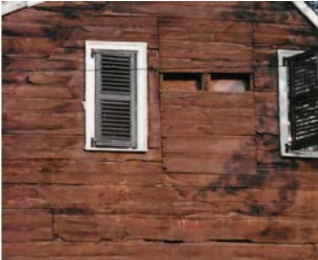
Figure 5d. - West gable during 2002 removal of weatherboard. Note the large square patch behind the chimney (Bierce Collection).
