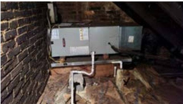
Figure 20e. - Air Handline Unit System - 1
