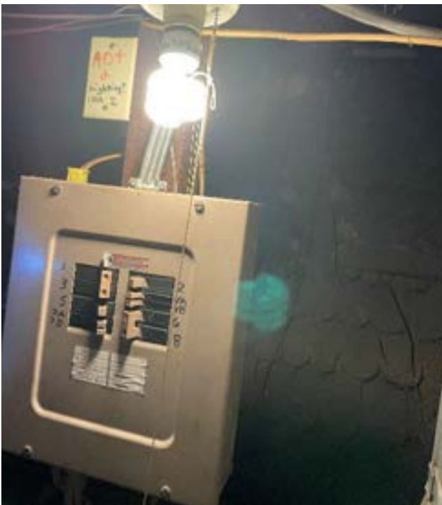
Figure 20u. - Light fixture in the Attic
