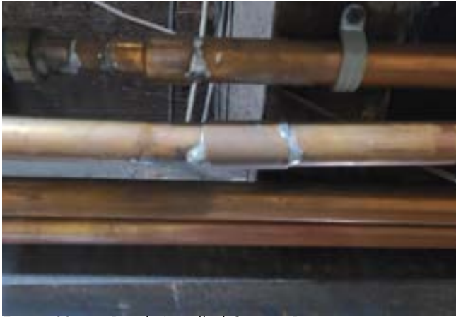
Figure 20an. - Poorly Installed Copper Piping
