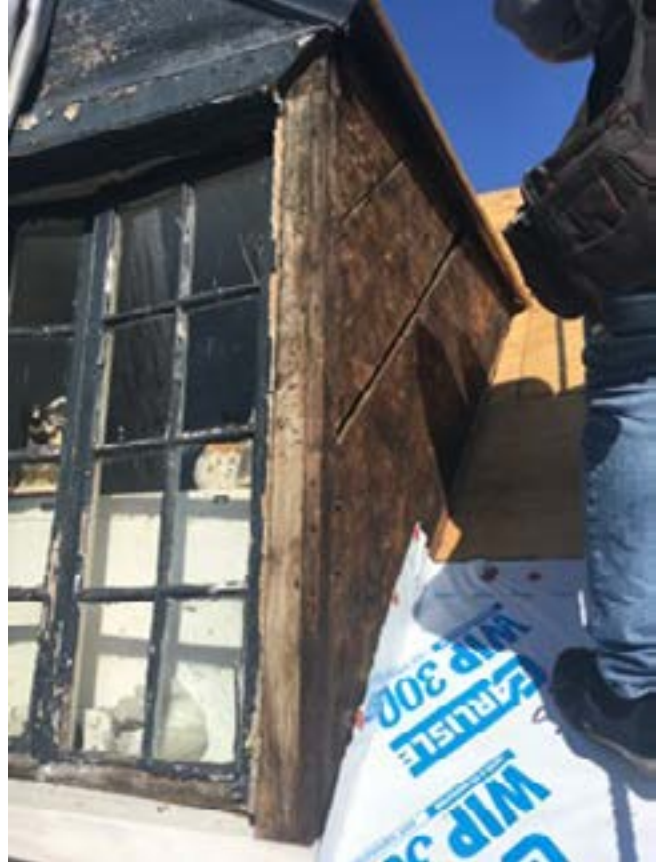
Figure 15d. - Typical south dormer showing original diagonal sheathing that shows no signs of any covering other than shingles.
