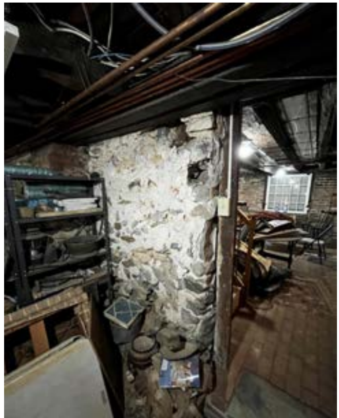
Figure 19d. west jamb of the door between the 1784 and 1774 sections looking south (Room 104)
