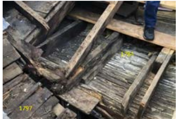
Figure 5b. - Roof and joists at NW corner of 1784 Addition during roof repair of 2022 looking SW. Note the modern sisters flanking the badly deteriorated joist to right at the former corner chimney location, making it hard to find evidence of a chimney. According to contractor Hank Handler, during the 2022 repair he saw charred debris at the next joist to the west, possibly indicating a chimney there [Al Cox photo, Exterior Restoration PowerPoint, Historic Alexandria, Alexandria VA].
