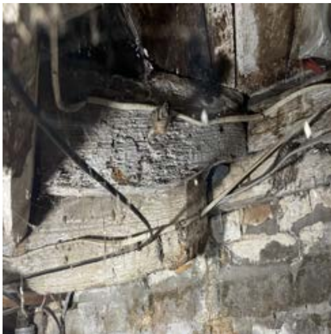
Figure 5a. - Junction of diagonal framing for the chimney with the sill in the NW corner of the 1784 addition.
