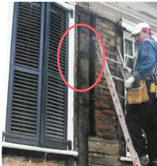
Figure 8f. - South front during restoration in 2002. The location of the bevel for the door head can be seen on the intermediate post that originally served as the door post near the top rung of the ladder (Bierce Collection, Historic Alexandria).
