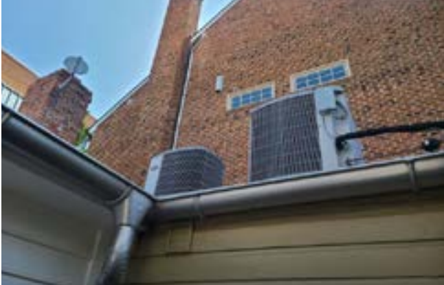
Figure 20g. - HVAC System 2&3 Air Cooled Condensing Units
