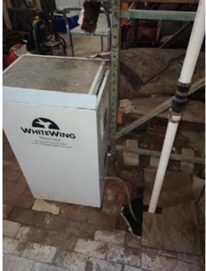
Figure 20p. - Dehumidifier Adjacent to Sump Pump
