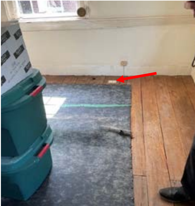
Figure 20ag. - Floor Receptacle in the Chamber
