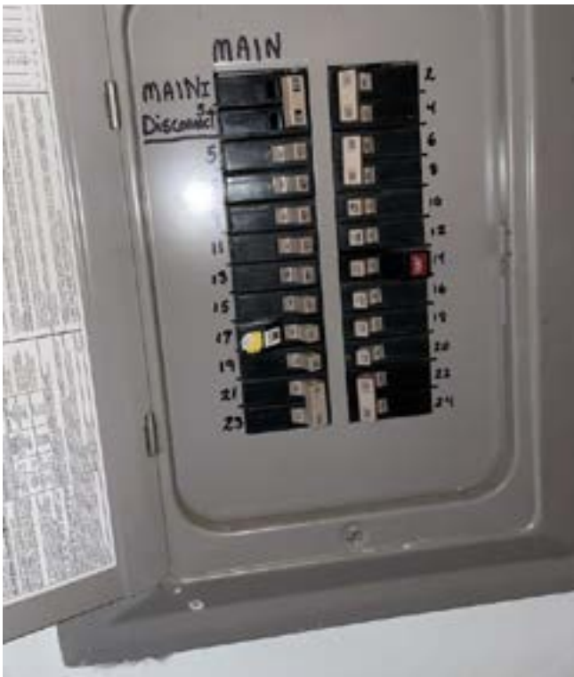
Figure 20y. - Panelboard Located in Corridor 112
