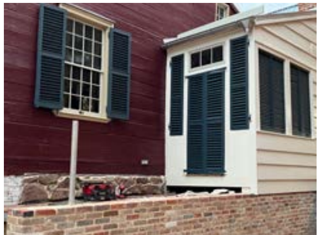
Figure 7u. - Reconstruction of east porch in 2022, Before (above) and After (below), Al Cox, Historic Alexandria, Alexandria VA. Note the modern but historic-style gutter in place before restoration and the restored gutter afterwards.
