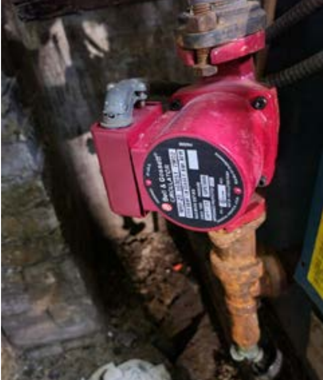
Figure 20n. - Radiant Heating Circulation Pump
