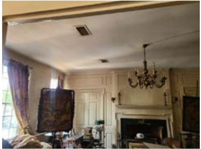
Figure 20i. - HVAC Registers in the Living/Parlor Area (Rm 104) Ceiling
