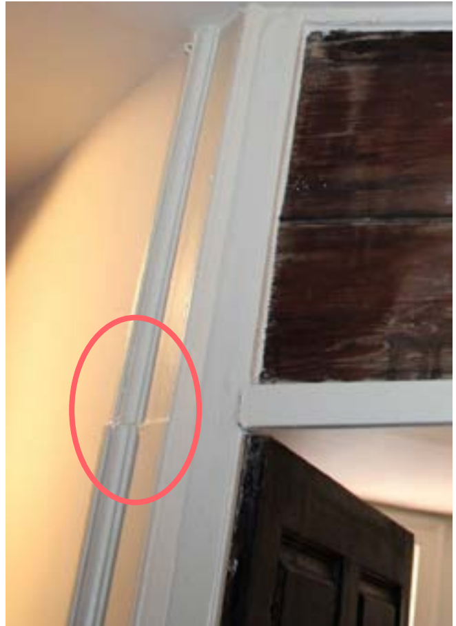
Figure 8n. - North jamb of the door from the NE Chamber to the passage looking NE. Note the 1784 door jamb to the left with a seam at door head height. It was extended to the ceiling when the door was reinstalled at a 45 degree angle.
