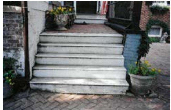
Figure 7t. - East entry before the steps and retaining wall were restored in 2022 (Bierce Collection, Historic Alexandria).
