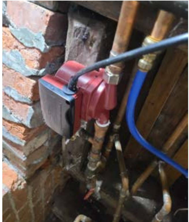
Figure 20ar. - Domestic Hot Water Inline Recirculation Pump
