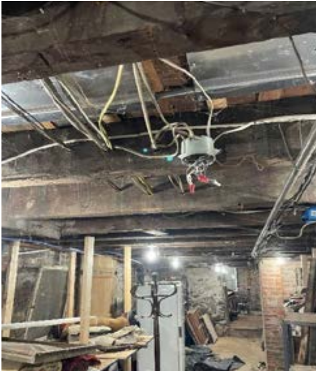
Figure 20ad. - Exposed Wiring in the Cellar
