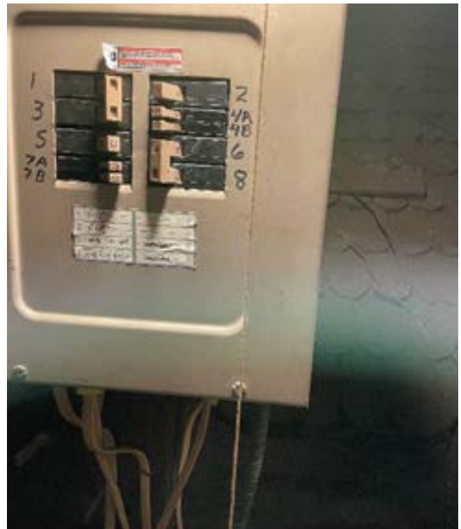
Figure 20aa. - Panelboard Located in the Attic
