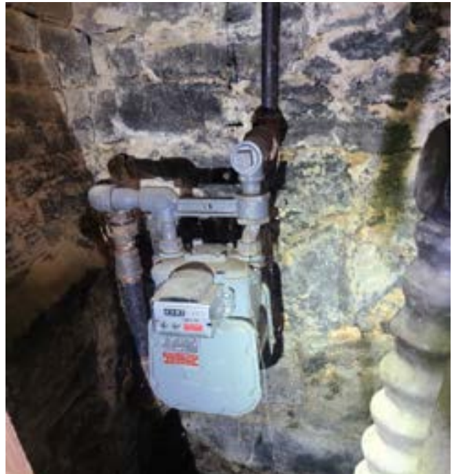
Figure 20ap. - Existing Natural Gas Meter in Cellar
