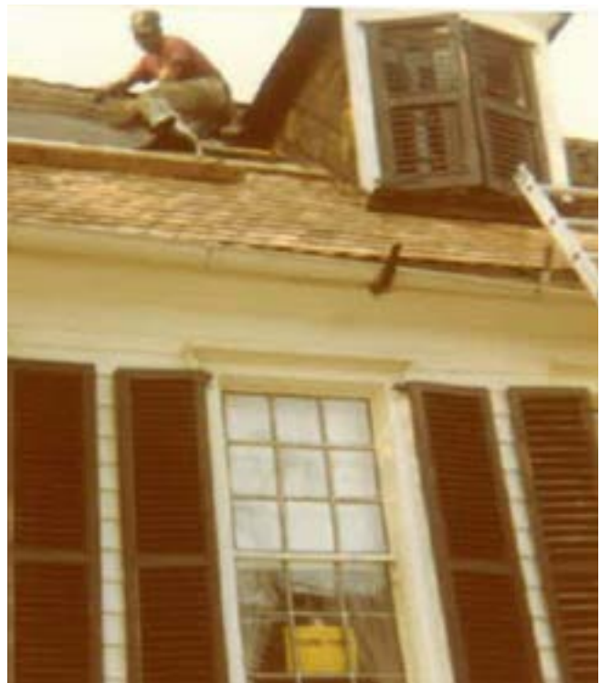
Figure 10j. - Reroofing the south slope of the 1774 roof shown in 1981 photo [Family Collection].
