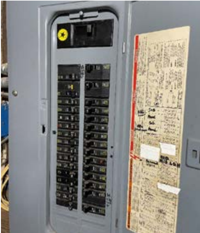
Figure 20x. - Main Panelboard in the Cellar
