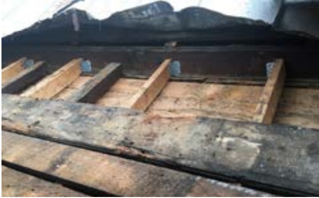
Figure 7g. - The west roof was uncovered during the replacement of the roofing in 2021. The nearly square rafters were resting on a ledger nailed to the fascia board (Al Cox).
