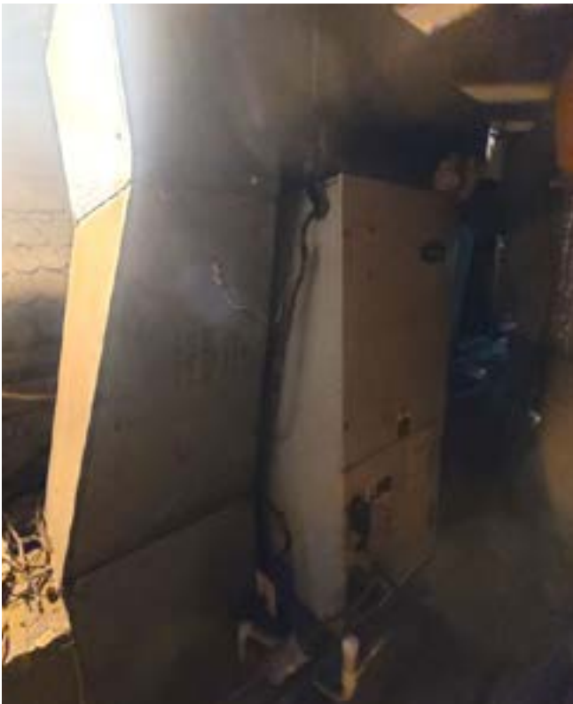
Figure 20h. - Existing Air Handling Unit - System 2 in the Attic
