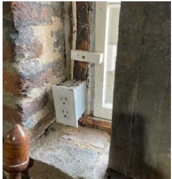
Figure 20af. - Receptacle in the Cellar
