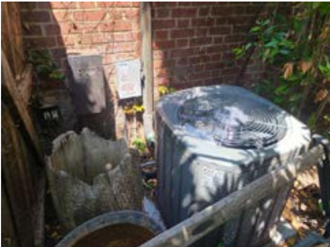
Figure 20d. - HVAC System 1 Air Cooled Condensing Unit
