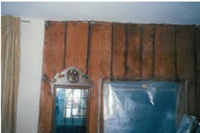
Figure 8m. - 2002 photo from the south of the vertical board partition between the NE Chamber and the adjoining closet, showing vertical board partition, original door location with the door and trim removed (Bierce Collection, Historic Alexandria).
