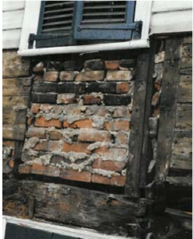
Figure 8c. - South front during restoration in 2002 showing the added brick filling or nogging below the added window sill with the added window post to the right (Bierce Collection, Historic Alexandria). Alexandria.
