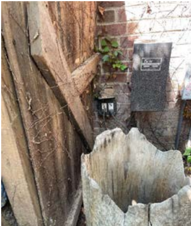
Figure 20ae. - Outdoor Receptacles with Improper Cover
