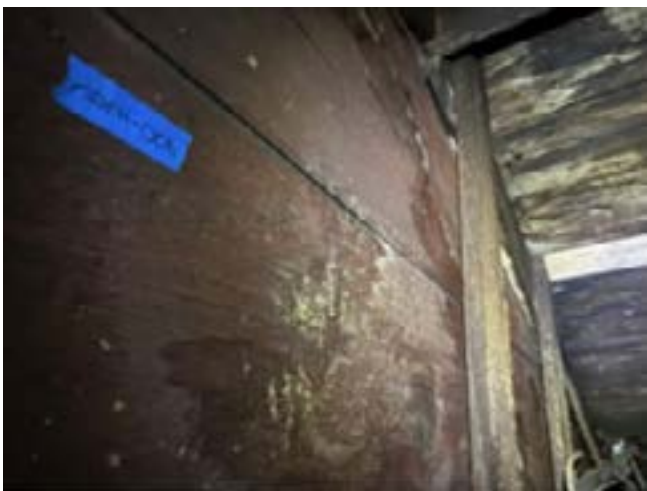
Figure 8i. - Original paint on the east exterior wall of the 1784 section seen from within the attic of the east extension of c1816.
