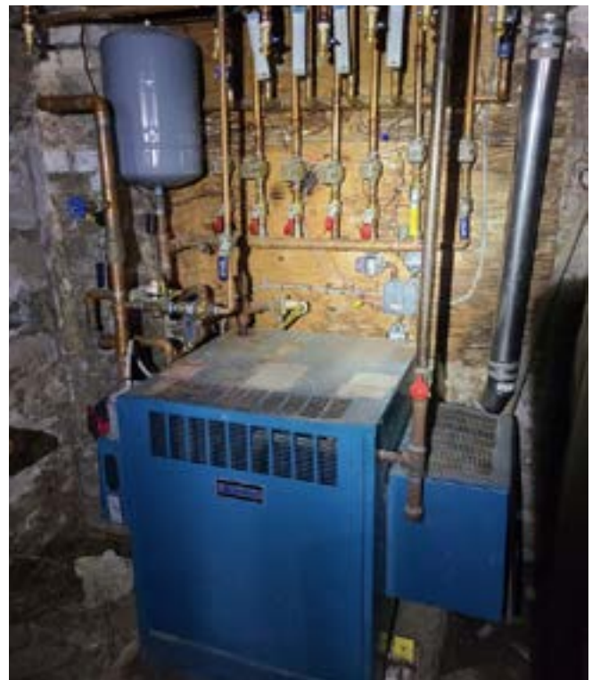
Figure 20m. - Hot Water Boiler in the Cellar
