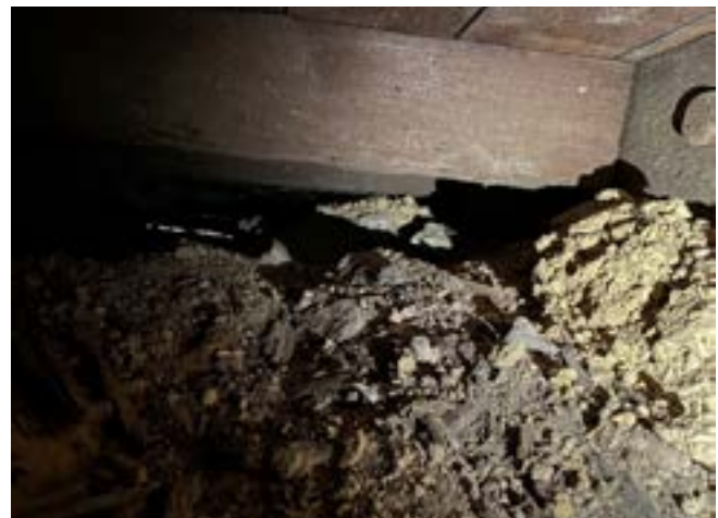
Figure 19n. Crawl space below the 1816 Extension looking at the east side of the sill of the 1784 Addition showing peg.
