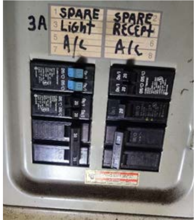
Figure 20z. - Panelboard located in Attic above Service room (Rm 114)
