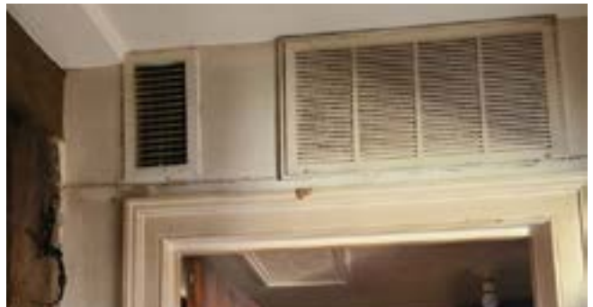
Figure 20j. - Supply and Return Grilles to HVAC System 3
