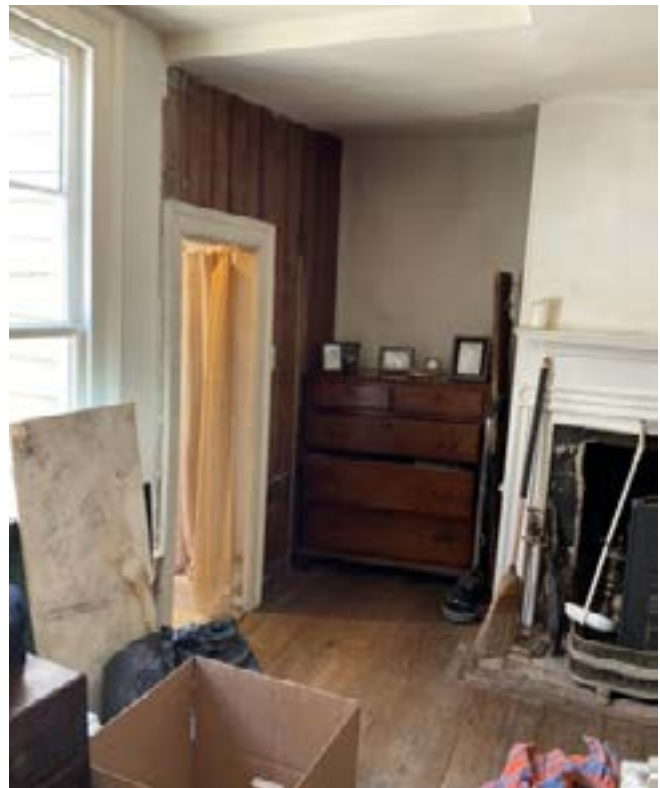
Figure 15p. - Room 107, (Northeast Chamber) northeast corner, looking NE. Note the door to the Closet (Room 108) in the board partition. See the repaired ceiling at the top.
