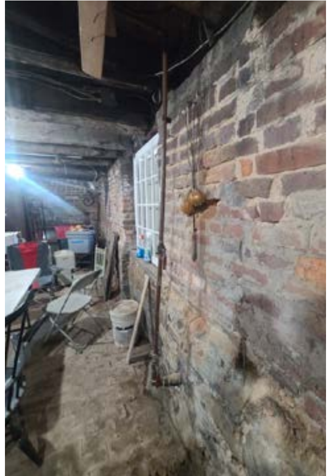
Figure 20am. - Incoming Domestic Water Service
