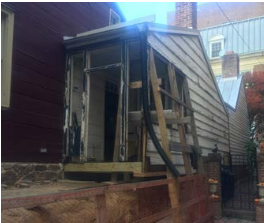
Figure 12e. - Al Cox, Photo of East Extension during repairs and insertion of new foundation, 2022..
