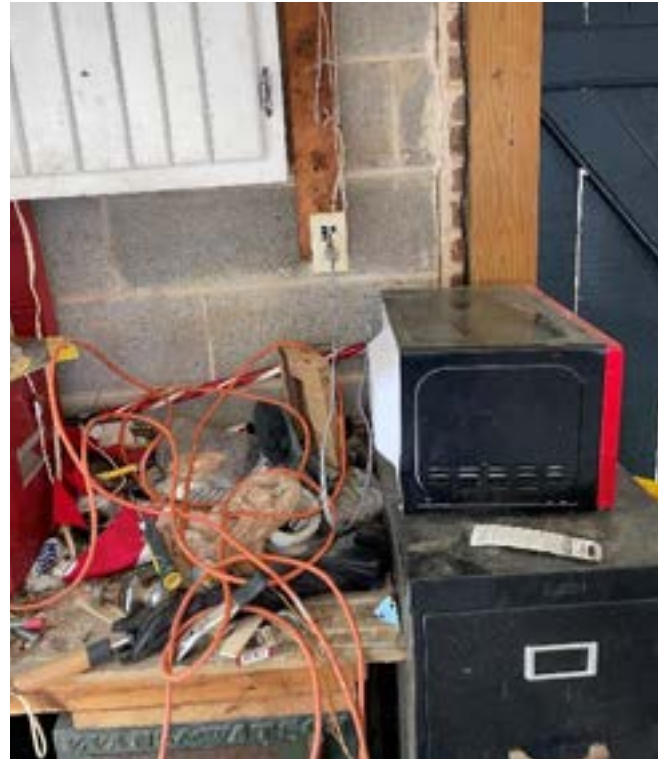
Figure 20ac. - GFCI Receptacle (Broken) in the Garage
